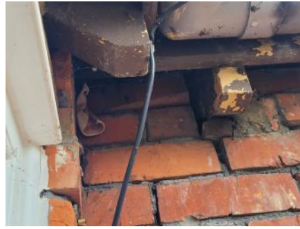
Photo 4: Loose brickwork around exposed rafter tail.
