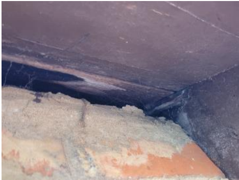
Photo 5: Gap between the wall top and roof.
