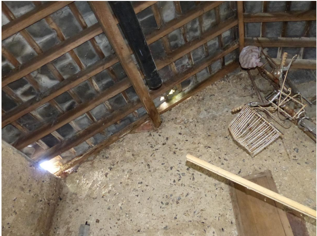
Figure 20: Interior of Outbuilding with unlined roof and visible gaps
