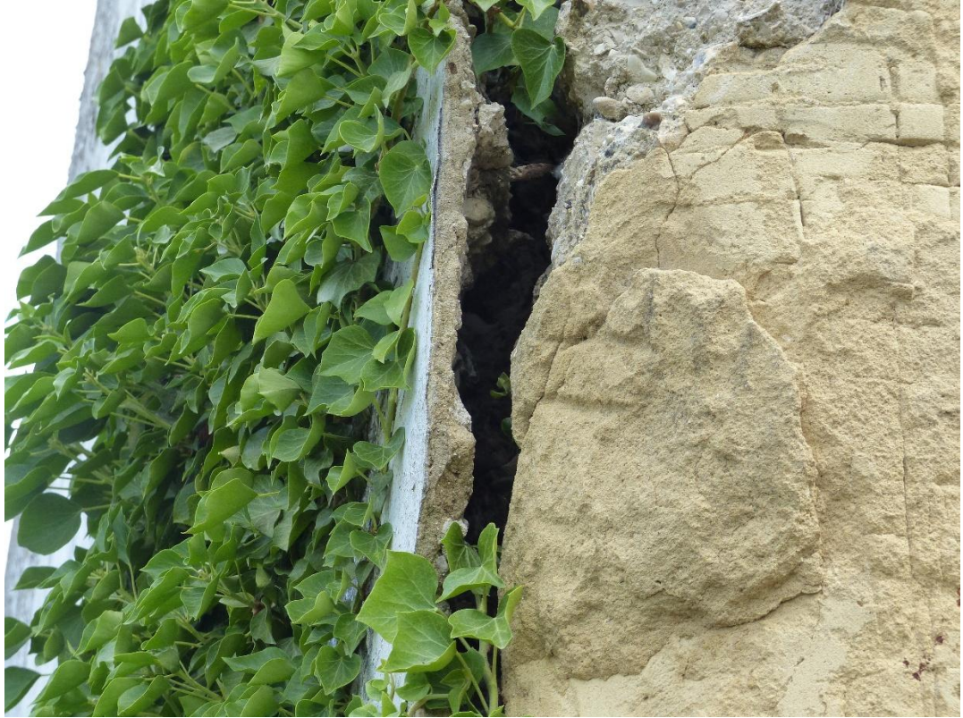
Figure 19: Gaps within exterior render on SW corner of Outbuilding
