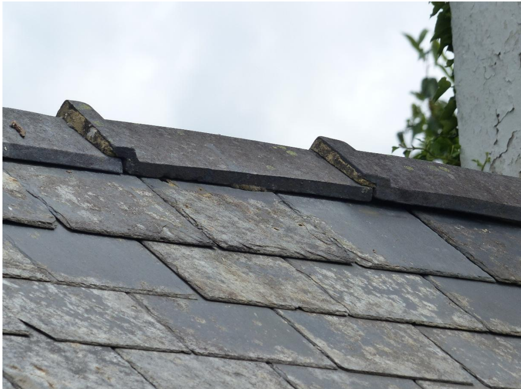
Figure 10: Missing mortar below ridge tile on western aspect extension
