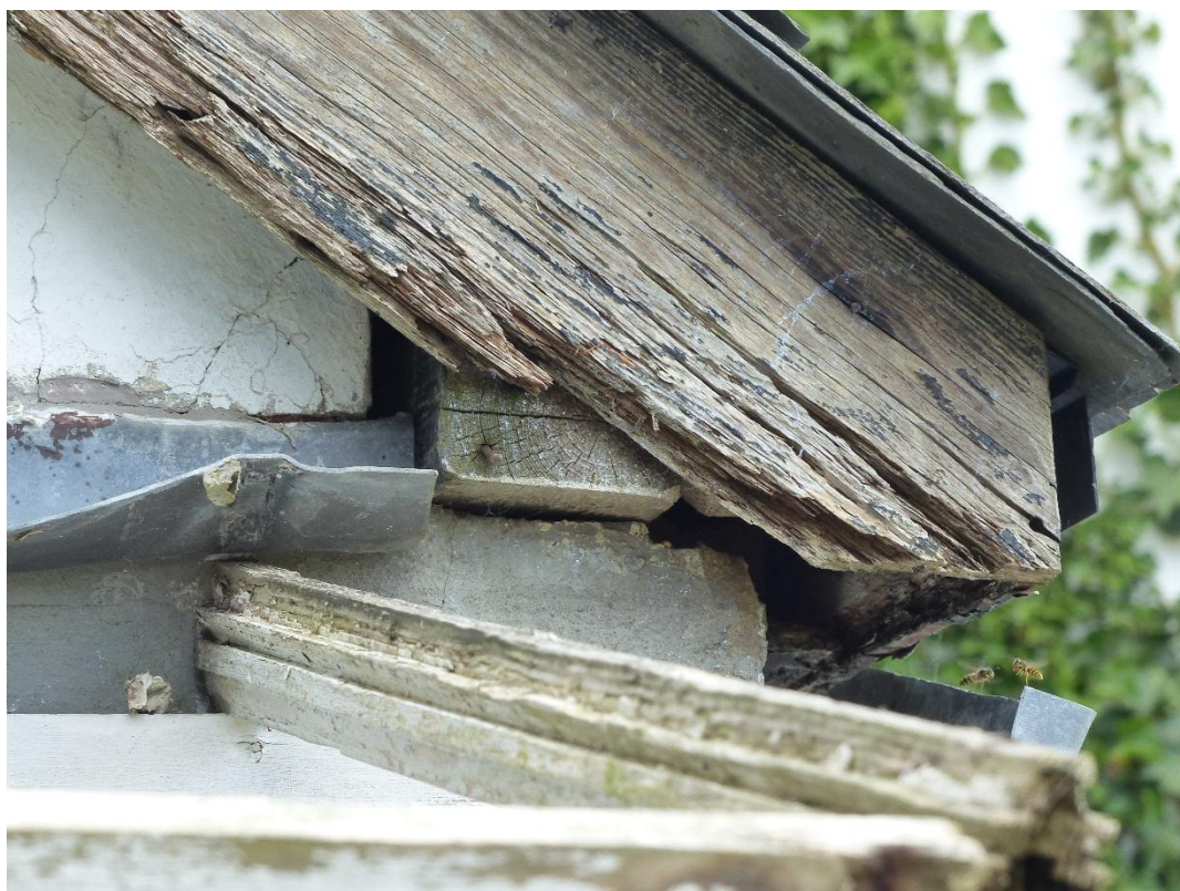
Figure 12: Gaps around barge boards and soffits on western aspect of extension
