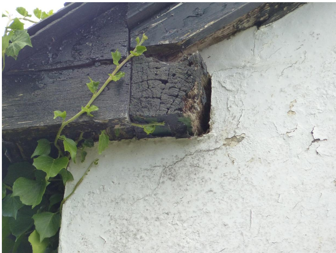
Figure 11: Gap alongside wall cap beam on western aspect
