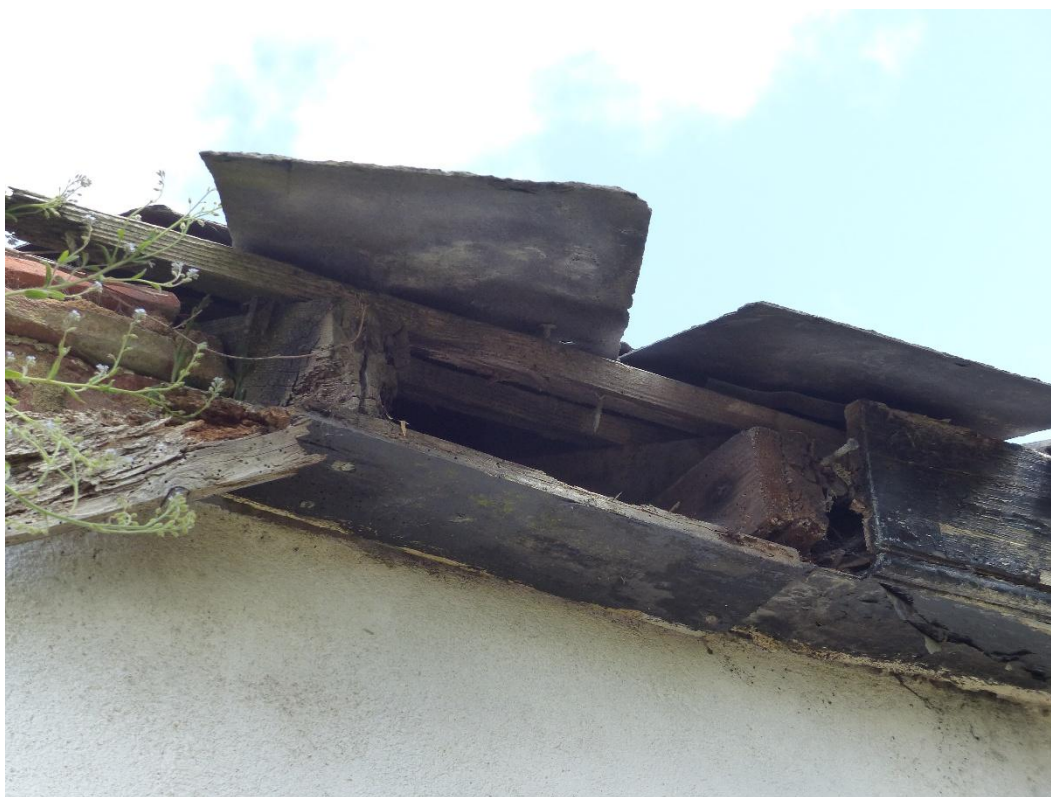
Figure 18: Gaps around eaves & slipped slates allowing access to building interior
