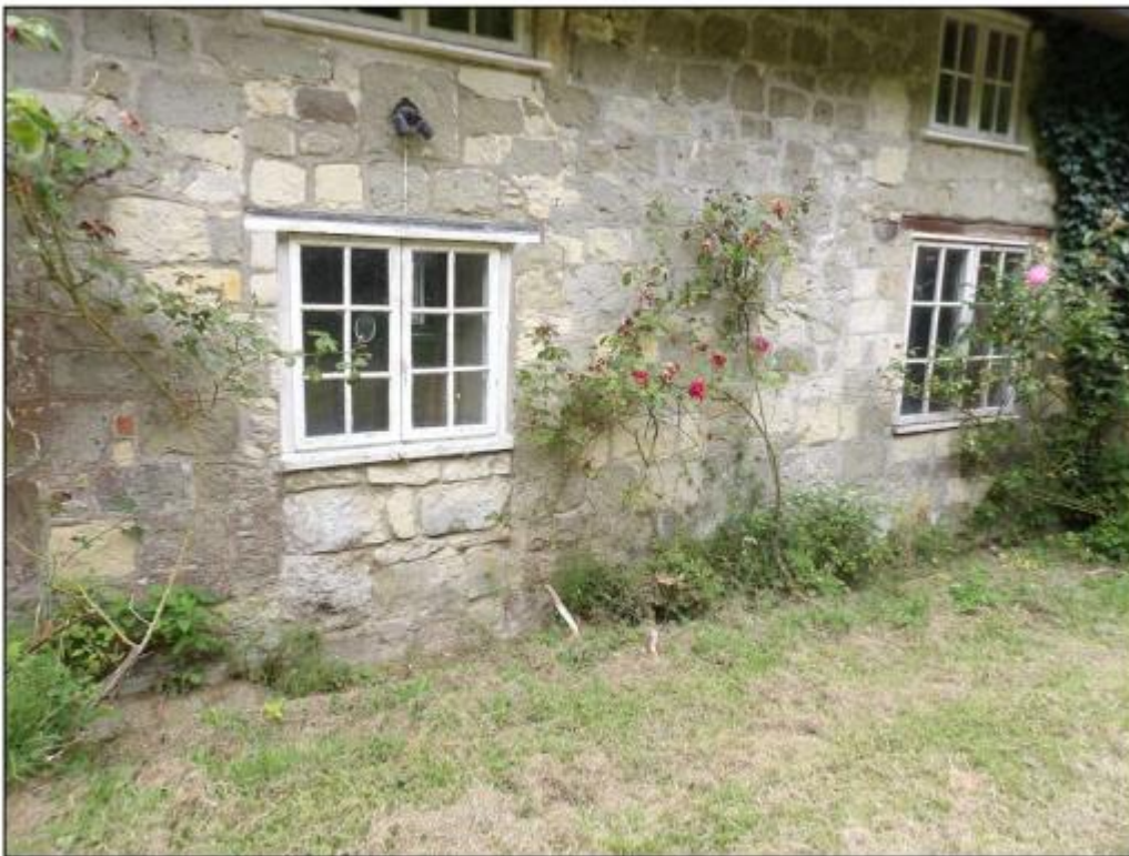
The principal elevation with the window replacing a former door. Notably the inserted window is smaller and the sill height also differs.
