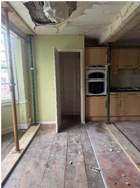
Cupped floorboards first floor. Feb26
