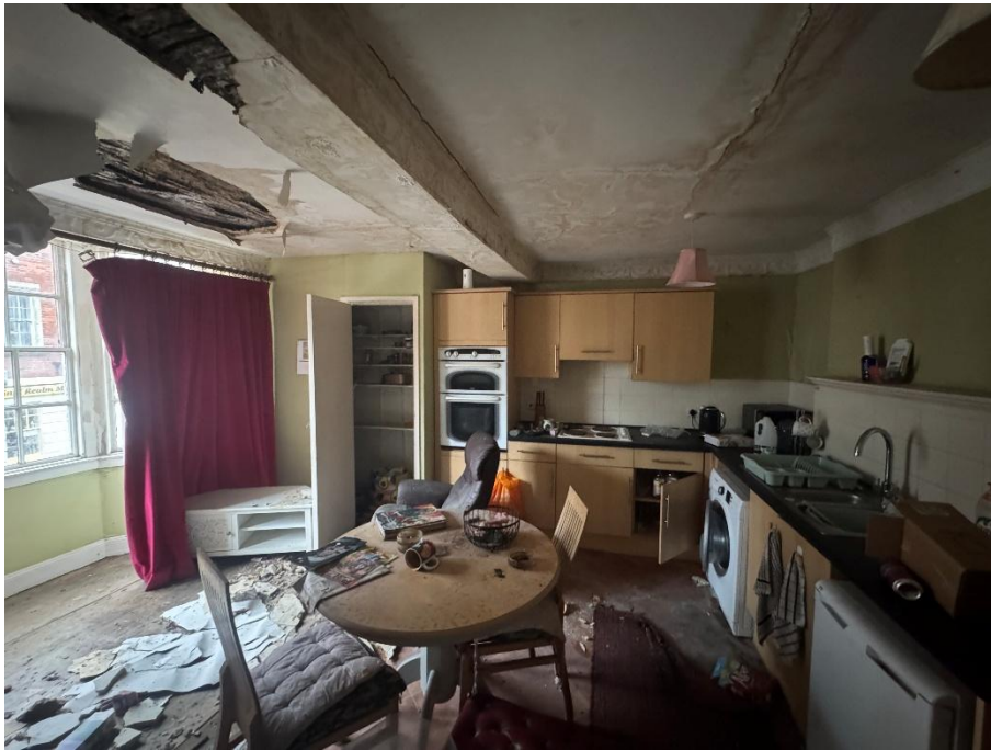
Ceiling damage first floor. Dec 25
