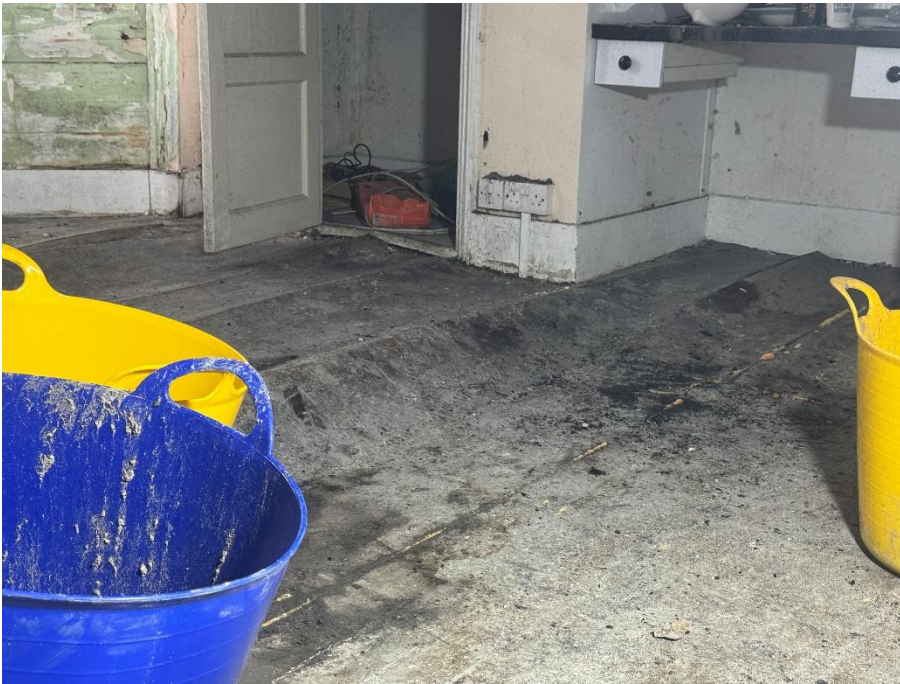
Damaged floorboards second floor Feb26
