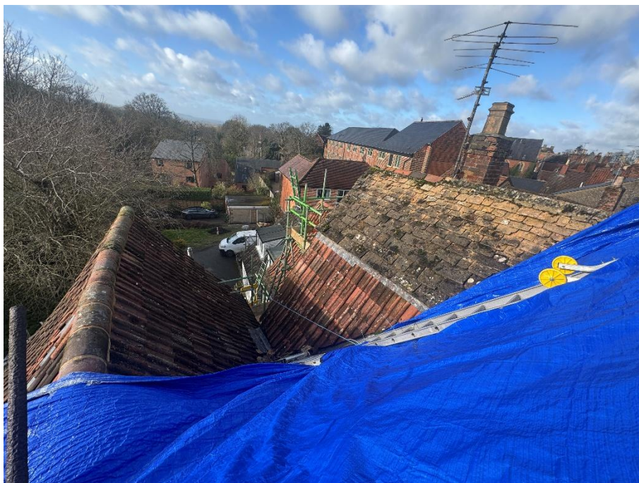
Right pitch- Part pantile, part stone slate roof to be replaced in stone slate
