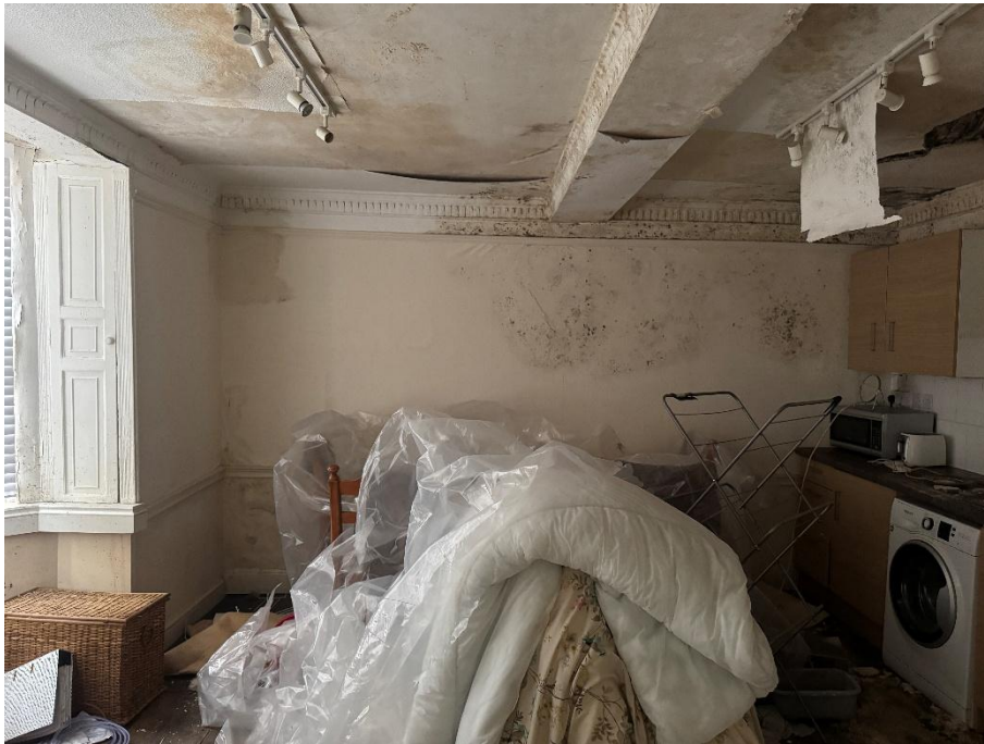
Ceiling damage ground floor. Dec 25
