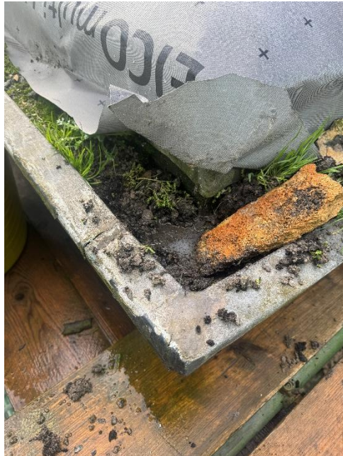
Failure at corners owing to expansion and contraction of lead around corners
