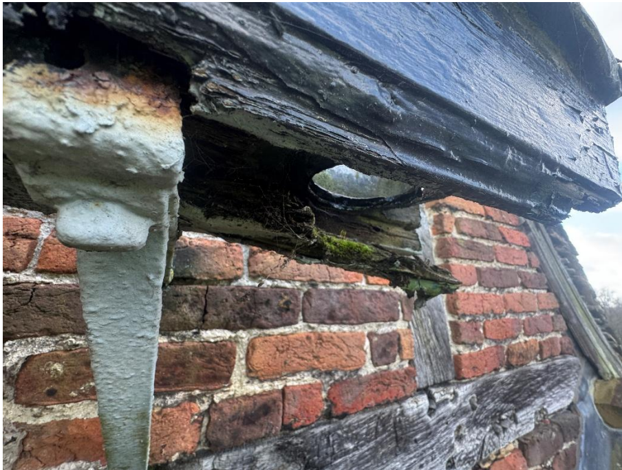
Failure of gutter west elevation
