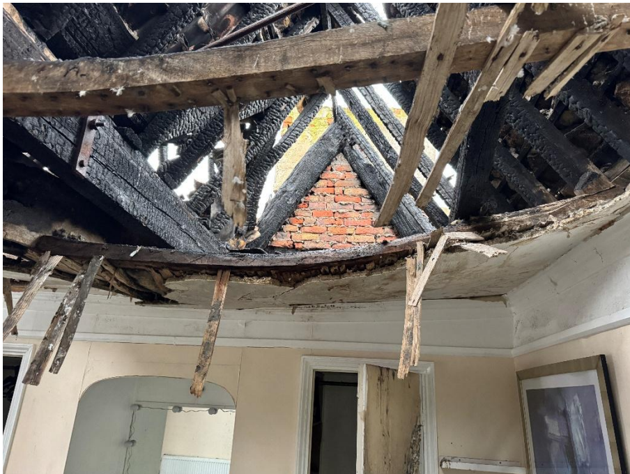
Ceiling damage second floor. Dec 25
