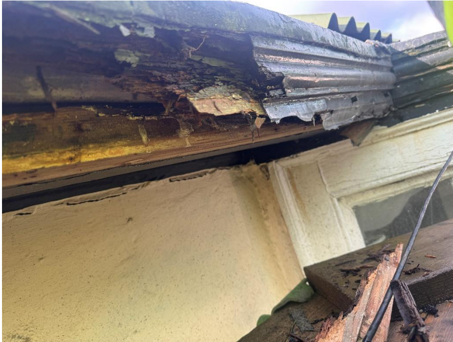
Failure of timber gutter east side of front elevation.
