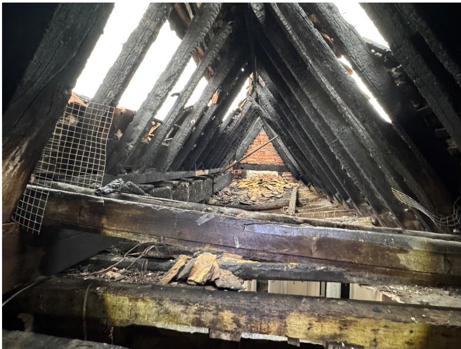
Fire damage to roof structure
