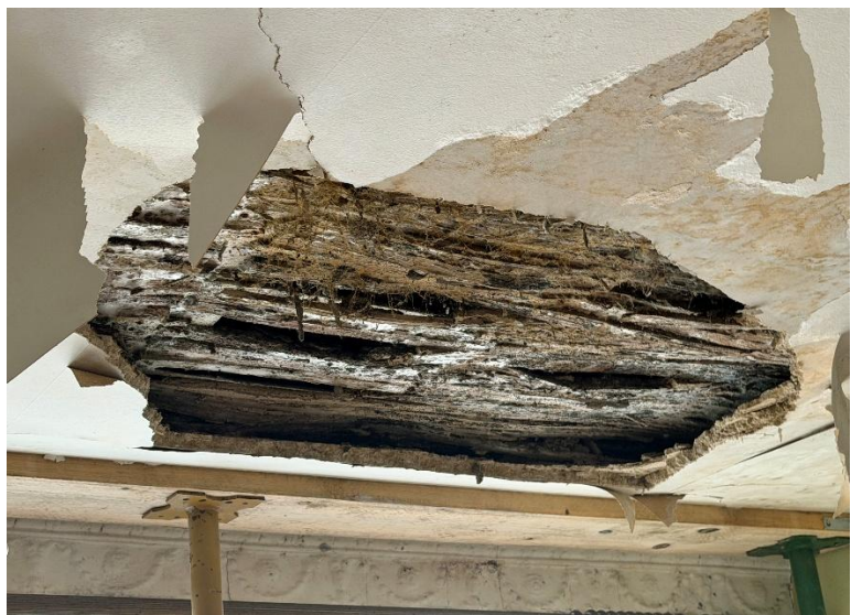
Fig.53 Laths exposed in ceiling
