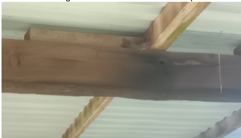
Photo 14. Showing swallow nest on roof timber of open fronted section of shed C
