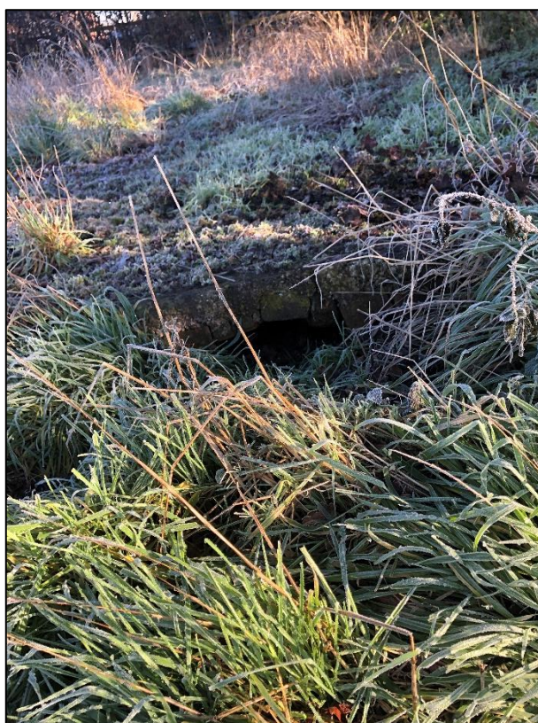
Photograph 1: Hole beneath a concrete platform in eastern section of Approved Development Site.
