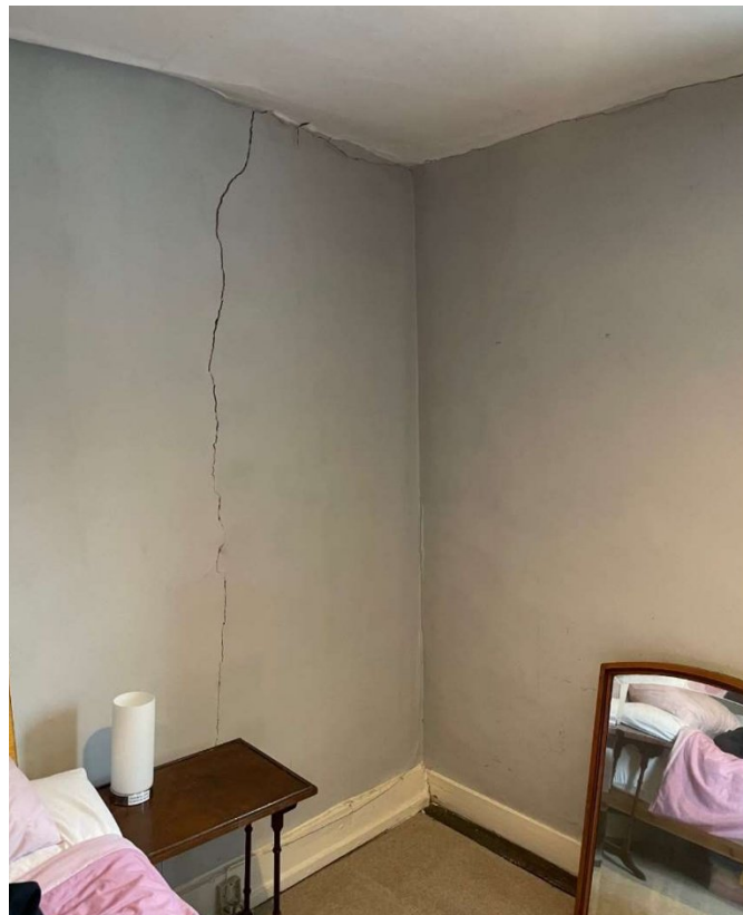
Image 9: Internal crack on 2 Pewsey Road
