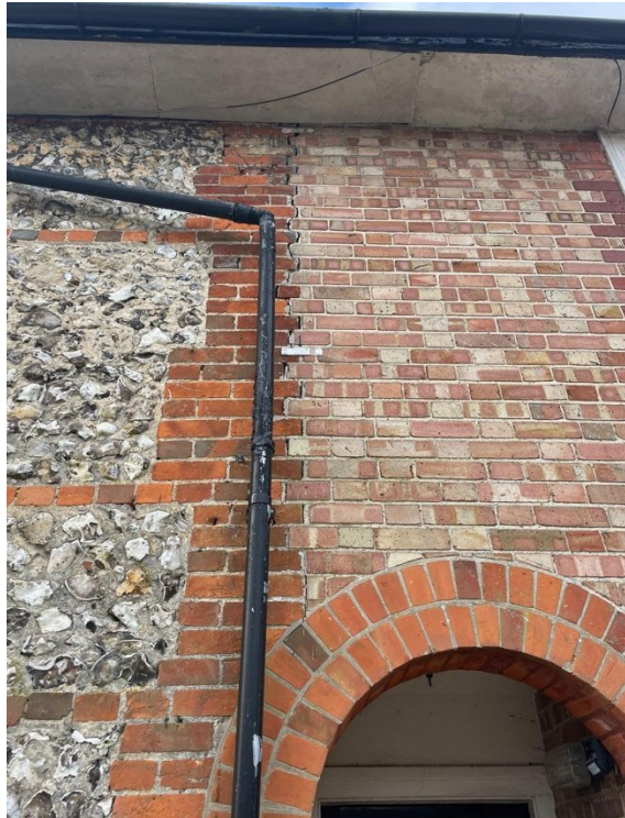
Image: 8 External crack on 4 Pewsey Road
