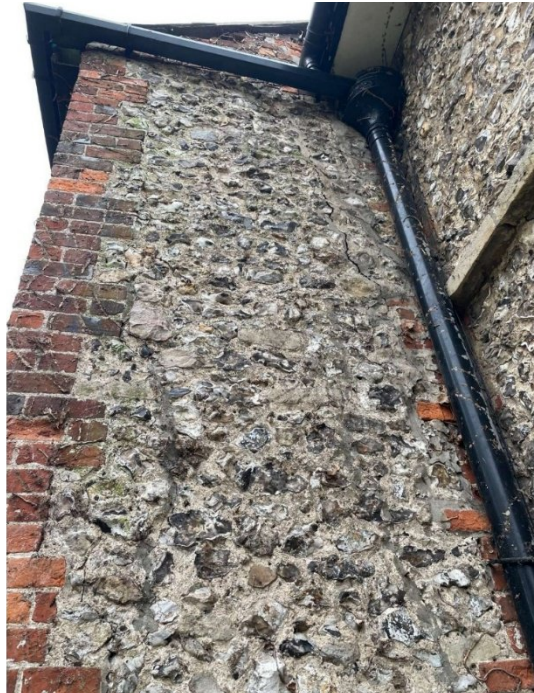
Image 7: Crack on 2 Pewsey Road flank return
