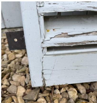
Sample of Damage to Shutters
