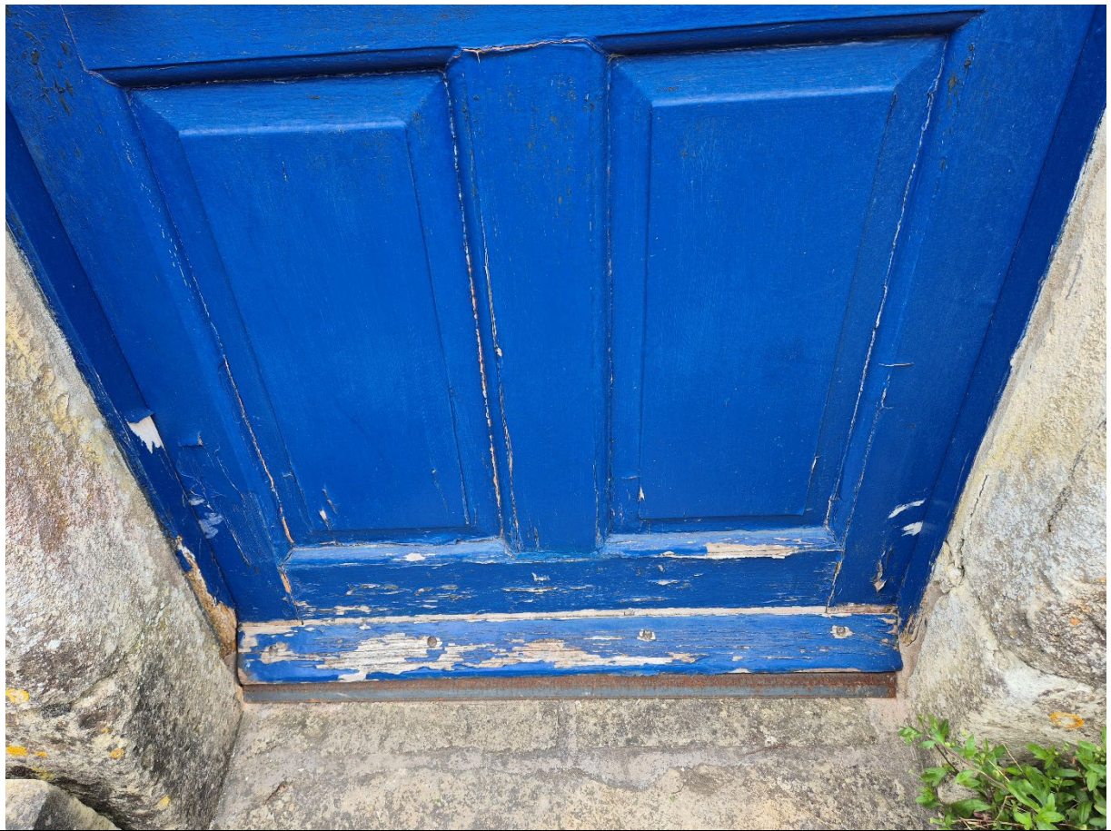
Fig 7: current condition of door (April 2026)
