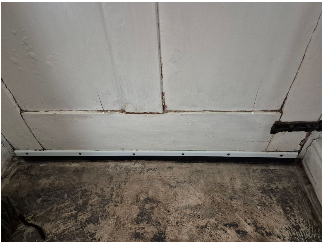
Fig 8: current condition of inside of door (April 2026)
