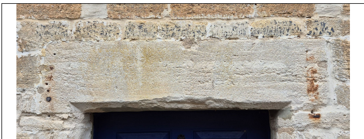
Fig 13: Surviving evidence of fixings for previous pentices. Note also deterioration of chamfered edge of stone
