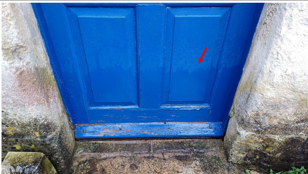
Fig 6: height of water splash back after typical rain shower (Nov 2024)
