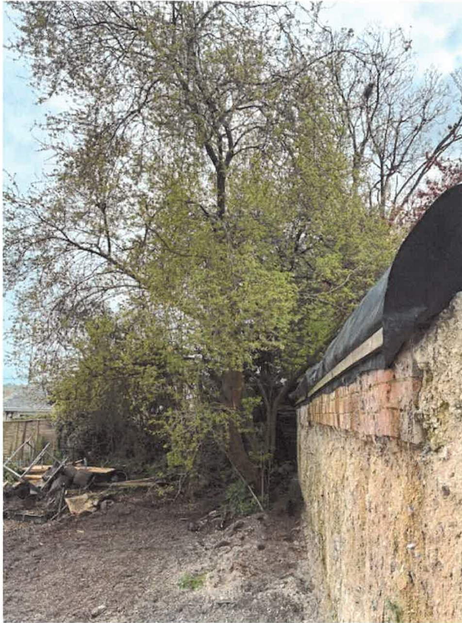
Plum Tree which is undermining the adjoining cob wall which is currently being rebuilt.
