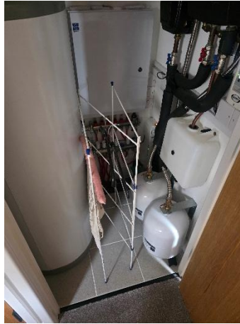
02 – Stair Landing Services Cupboard
