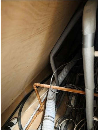
27 – Services to voids
