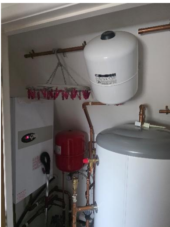
07 – Stair Landing Services Cupboard
