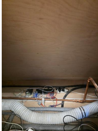
28 – Services to voids
