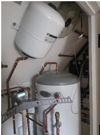
05 – Stair Landing Services Cupboard
