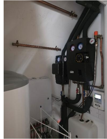
03 – Stair Landing Services Cupboard
