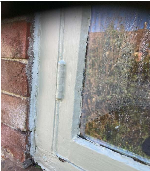
Detail lower left casement painted shut and rot to frame
