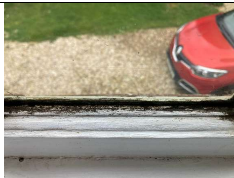
Note rot to bottom rail of casement
