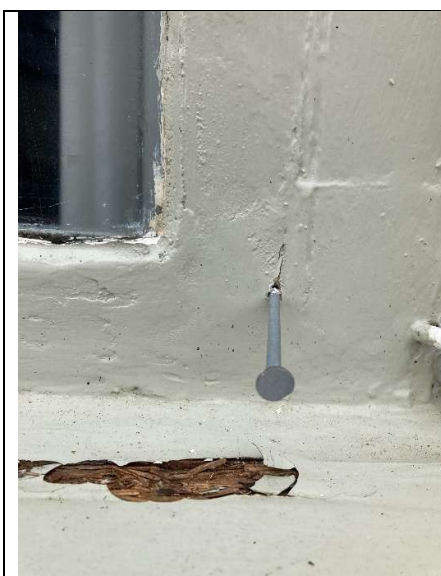
Rotten frame right side and note nail pressed into rotten frame
