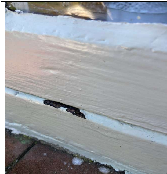
Window W1 centre of frame showing significant rot
