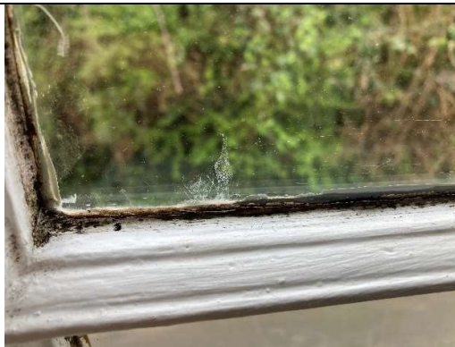
W4 note rot around casement frame
