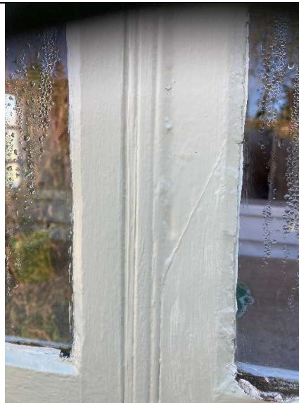
Centre mullion showing casement painted shut and rot to fixed casement frame
