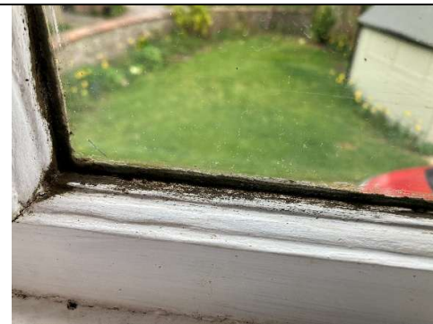
W1 note rot to casement
