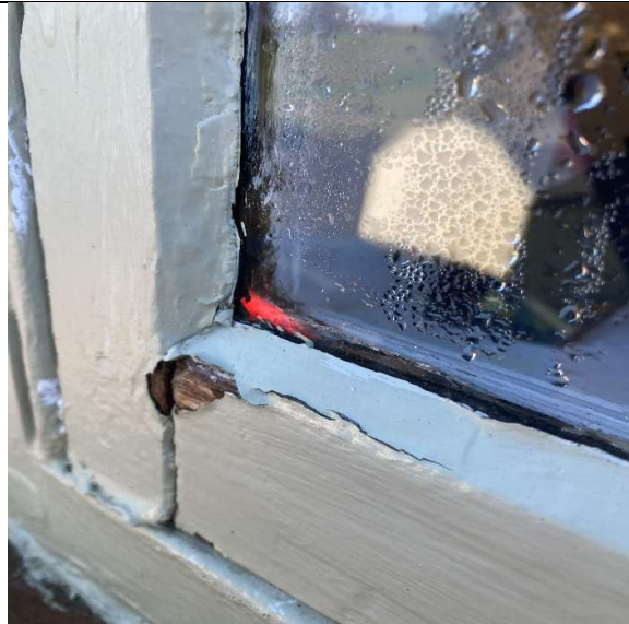
Window W1 left hand bottom corner- open casement joint and significant rot to frame
