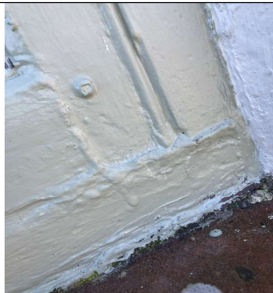
Window W1 right hand base of frame showing heavily filled and painted
