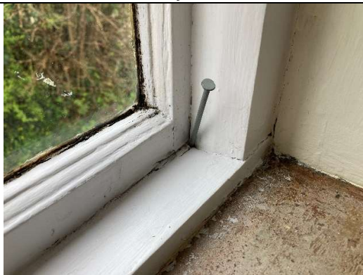
W4 Note nail pressed into rotten frame
