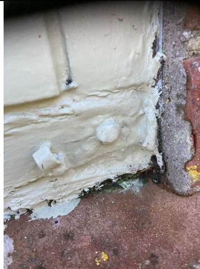
Detail on window frame lower left showing considerable rot to frame
