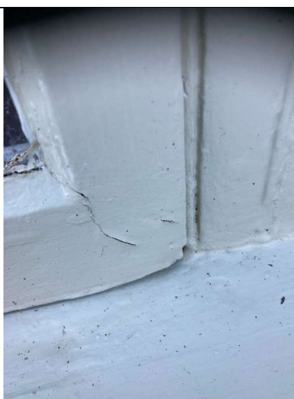
Cracked frame lower right side
