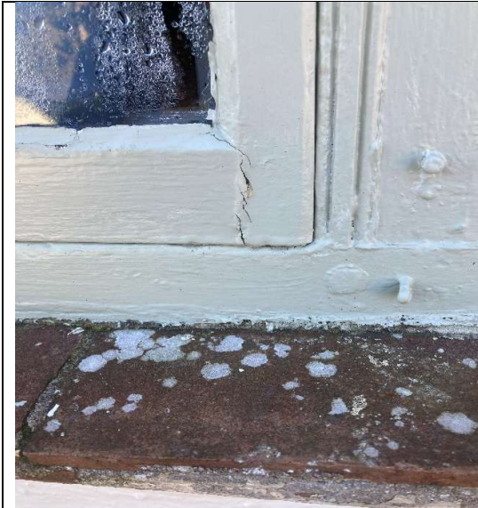
Window W1 Right hand bottom corner - Tiled cill – casement joints in poor condition
