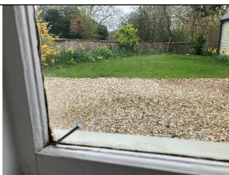
W2 note nail pressed into rotten casement frame
