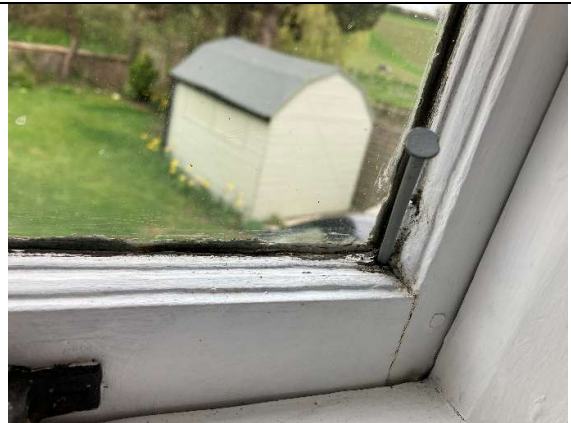
W1 note nail pressed into rotten wood in corner of casement
