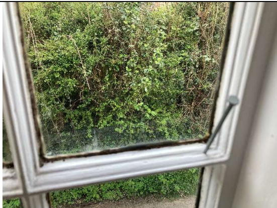
W4 note nail pressed into rotten glazing bar
