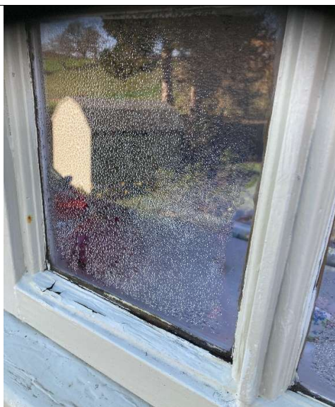
Significant rot to glazing bars
