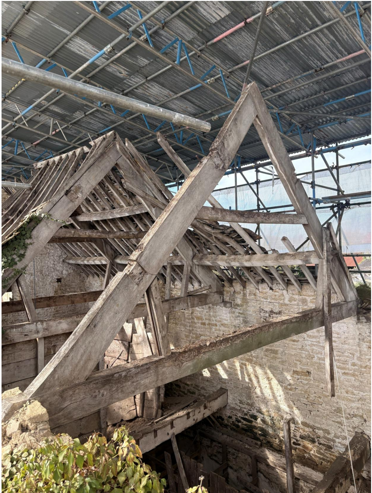
View of Eastern End Section of Roof – Note Missing (Collapsed) Roof Slates, Rafters and Purlins
