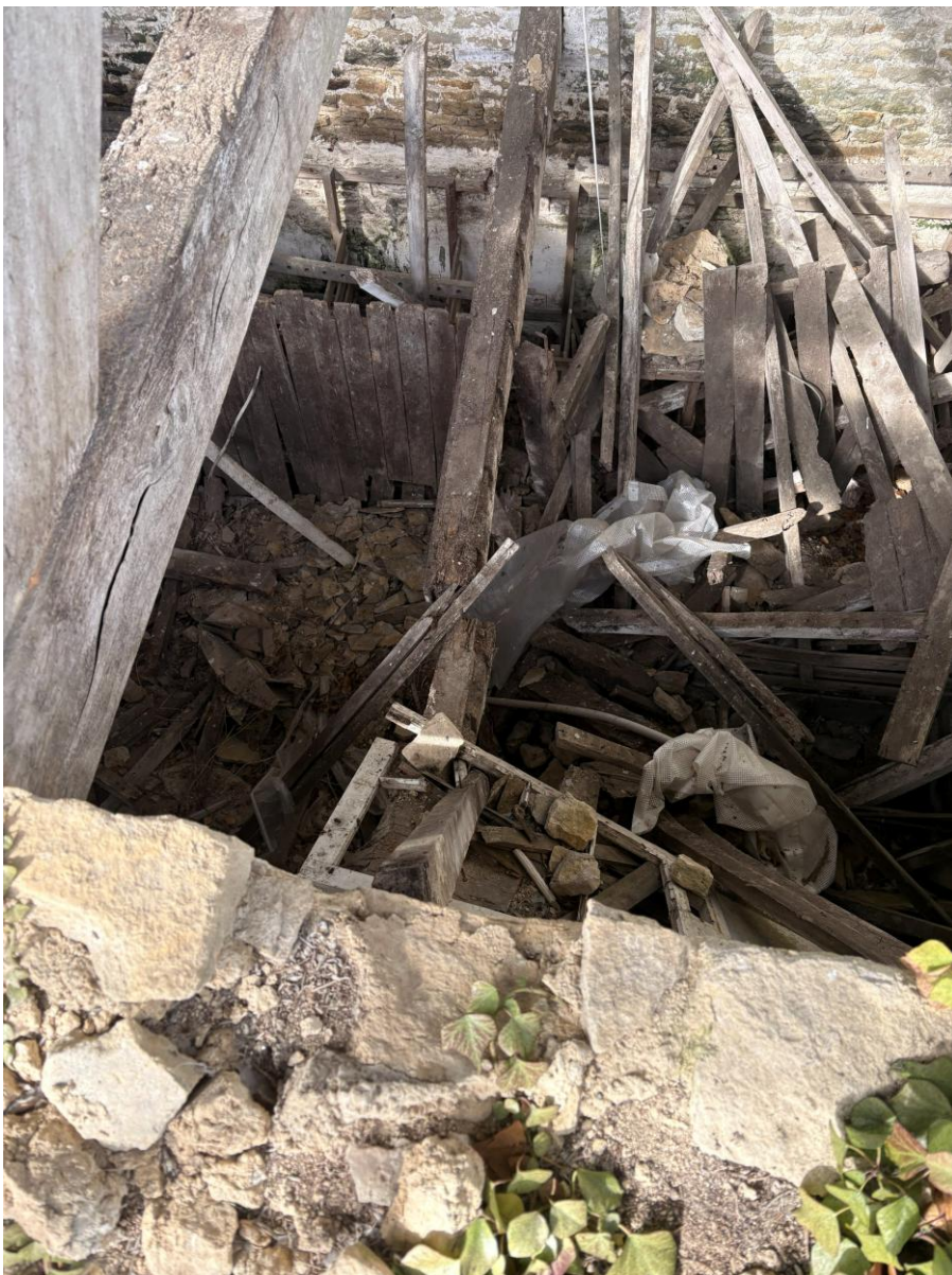
General View of Eastern Section Of Floor – Note Collapsed Beam and Missing Joists
