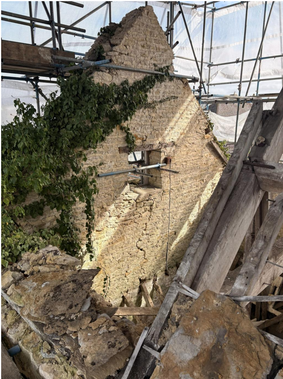
General View of Eastern Gable Wall – Note Vertical Cracking
