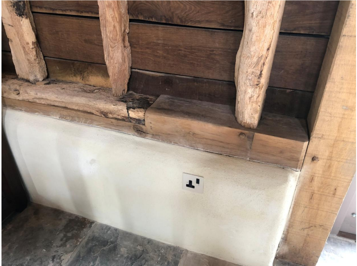
Possible Repair By Scarfing In of New Timber
