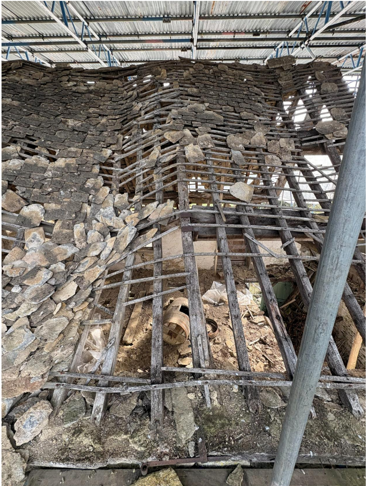
View of Mid – Section of The Roof – Showing Deformed and Partially Collapsed State of The Roof Fabric – Note The Dislodged ‘Rivers’ of Stone Slates
