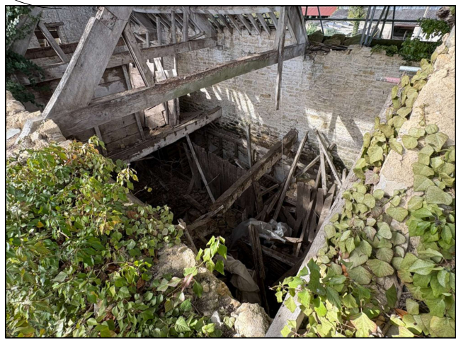
Significant amount of debris within the building, which appears to be roof structure material that has fallen in on the first floor that has further collapsed onto the ground floor. The build up of debris that is leaning on the external walls are starting to push the walls out.
