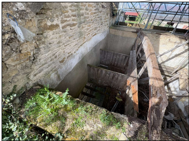
Debris within the building above passageway.
