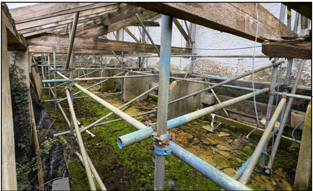
Debris within the lean-to building, which appears to be general stored materials.
