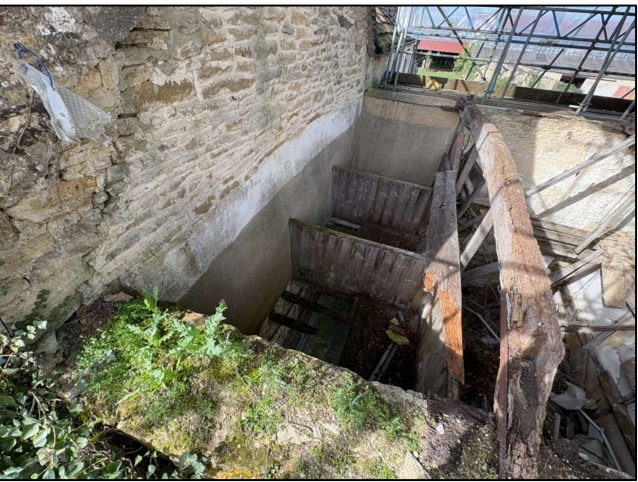
Debris within the building above passageway.
