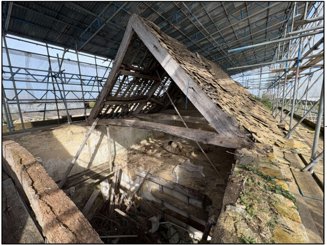
Significant amount of debris within the building, which appears to be roof structure material that has fallen in on the first floor. The build up of debris that is leaning on the external walls are starting to push the walls out with the first floor then eventually collapsing.
