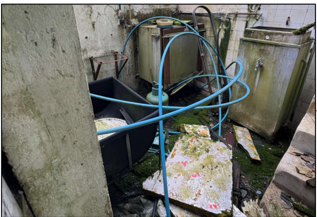
Debris within the lean-to building, which appears to be general stored materials.
