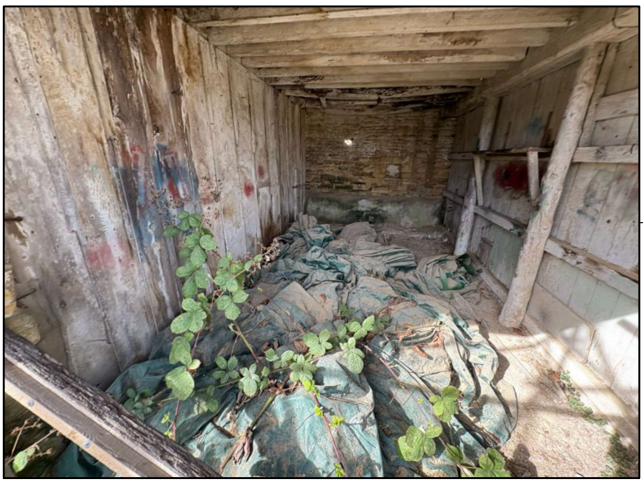
Significant amount of debris within the building on ground floor, which appears to be general stored materials.
