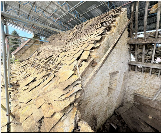
Section of existing roof with roof timbers and stone slates still in place. However, it appears that the roof timbers are starting to show signs of collapse.
