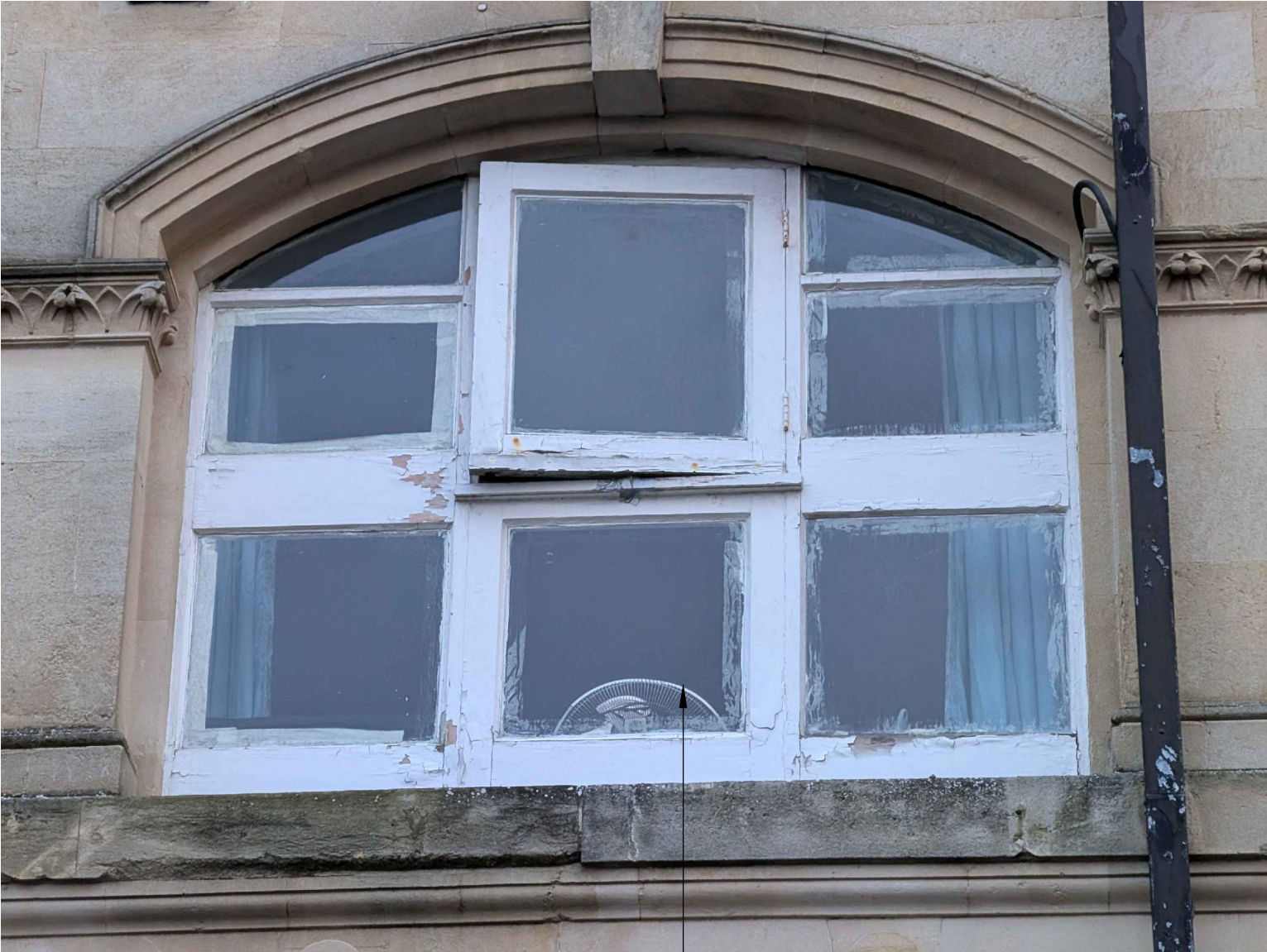
EXISTING NON-ORIGINAL REPLACEMENT WOODEN POOR STATE OF REPAIR, ROTTEN FROM THE OUTSIDE
