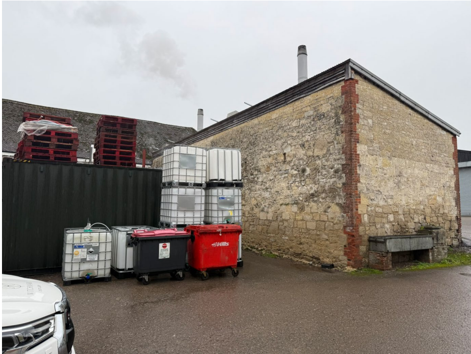
Photograph 3 – The siting of the external freestanding silos and vessels.
