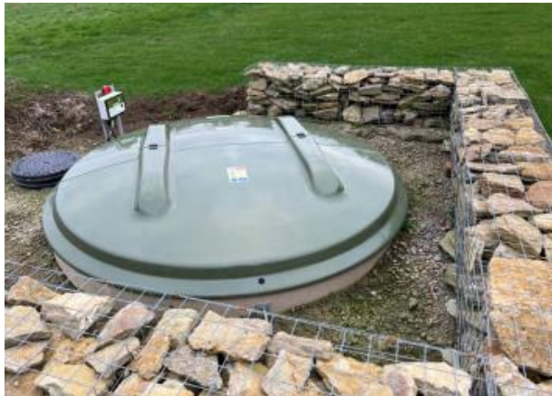
Figure 1: Sewage Treatment Plant
