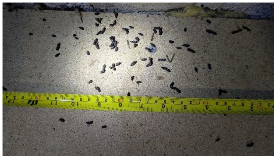
Photograph 13: Bat droppings noted at the northwest gable within the loft of B1.
