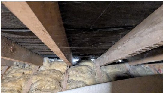
Photograph 11: An example of daylight noted along the eaves of the roof space of B1.
