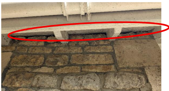
Photograph 7: An example of the gaps along the eaves of B1.
