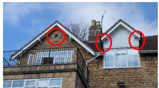
Photograph 8: Gaps around the dormer and ventilation feature noted on the southeast elevations of B1.
