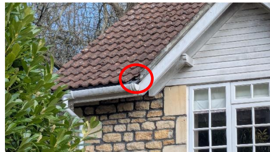
Photograph 6: Broken tile at the base of the dormer, southwest roof pitch of B1.
