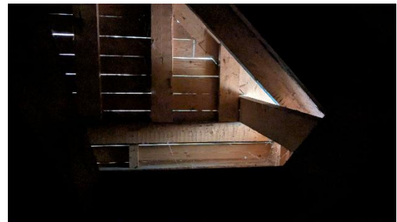
Photograph 12: Daylight noted from within the loft space, around the southeast dormer of B1.
