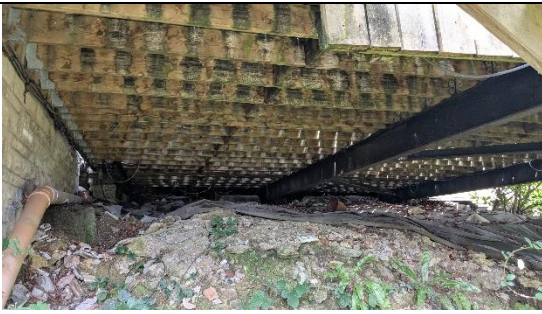
Photograph 9: The space under the northwest decking off B1.
