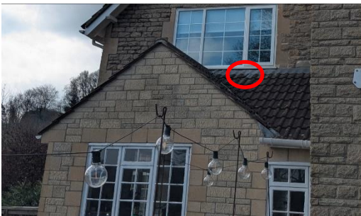
Photograph 5: The northeast extension of B1 with broken tile circled.
