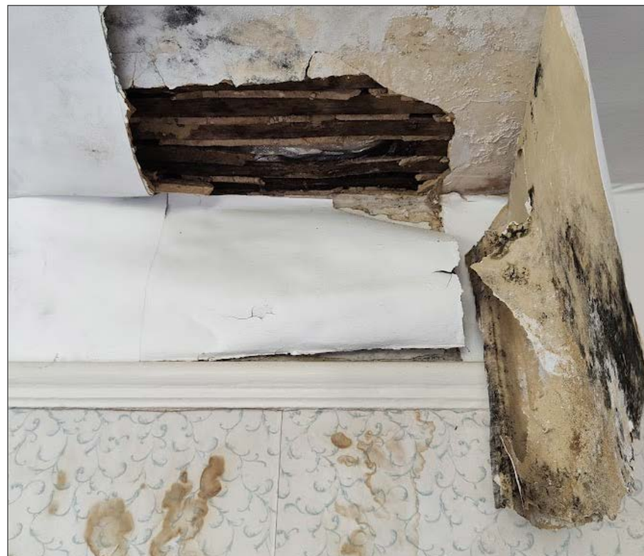
Figure 12: roof leaks causing internal damage
