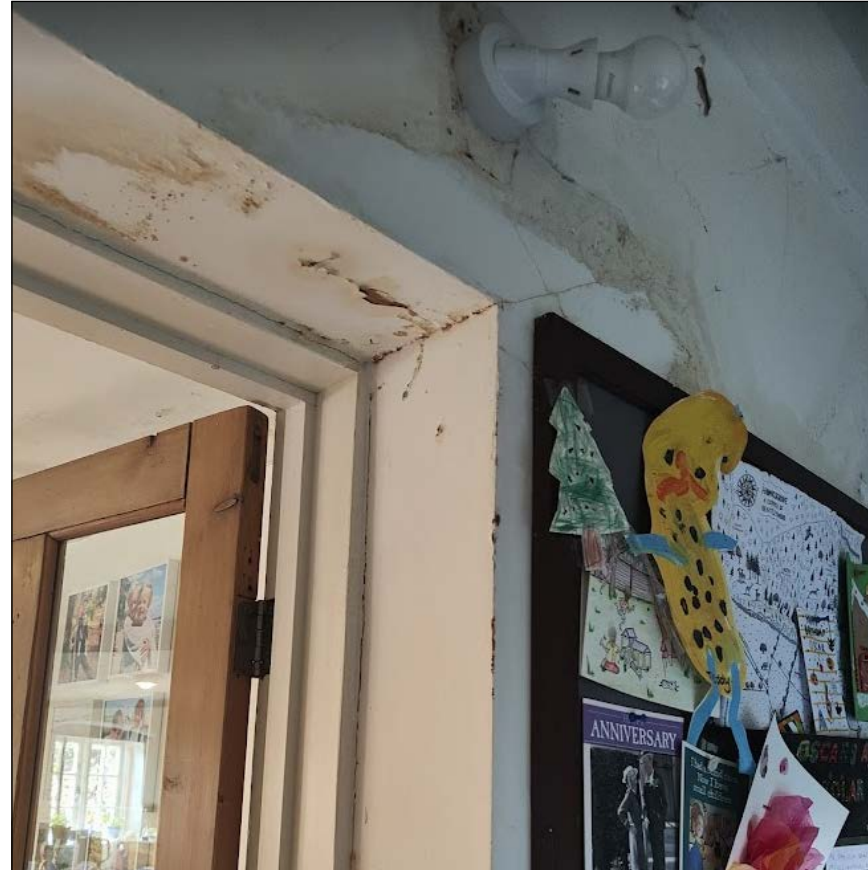
Figure 18: plasterwork damage from roof leaks
