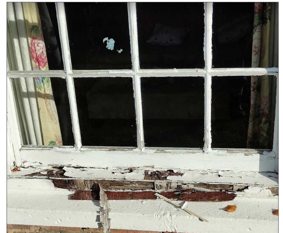
Figure 11: Required joinery repairs
