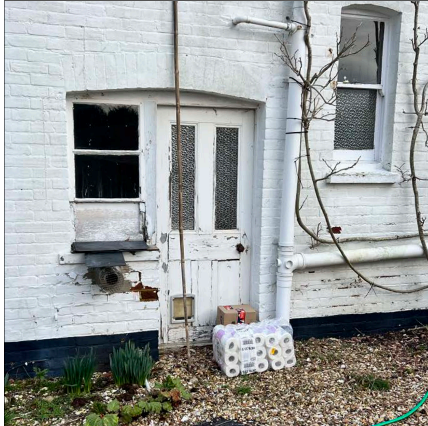
Figure 17: modern joinery to west gable to be replaced
