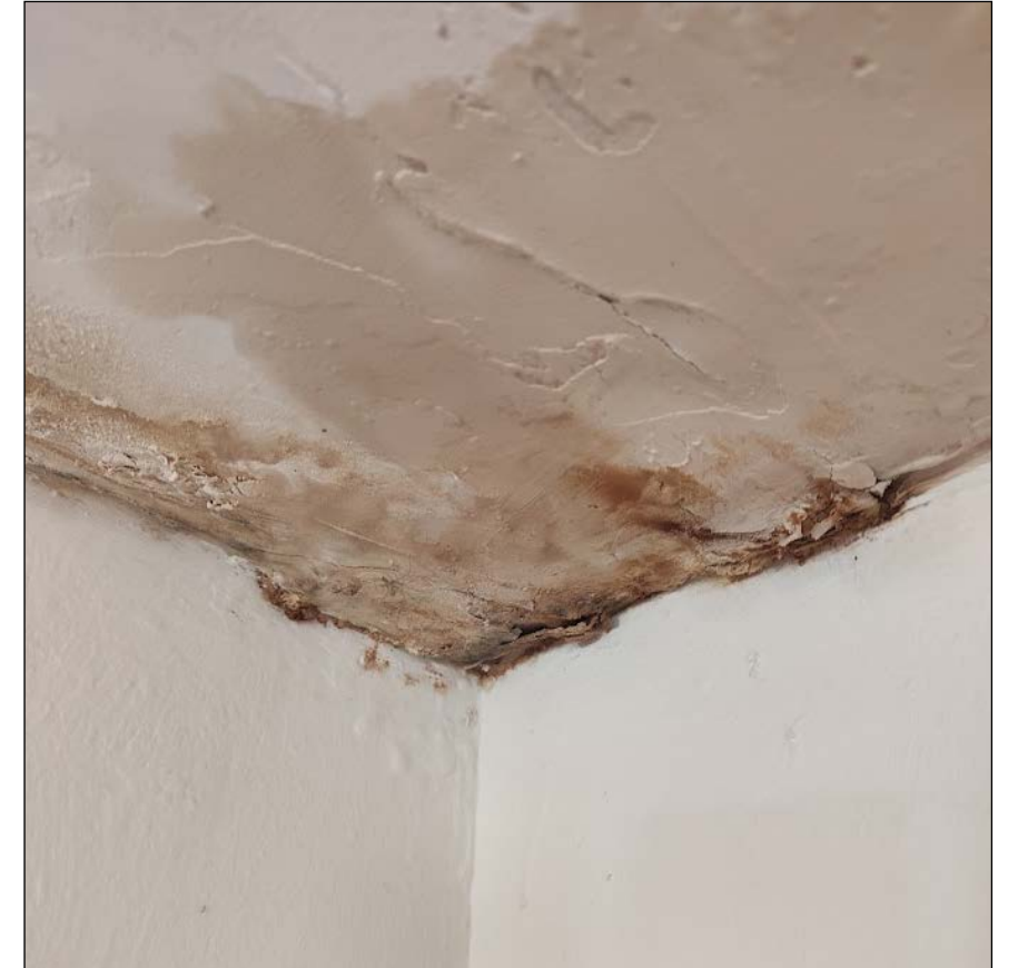
Figure 19: plasterwork damage from roof leaks
