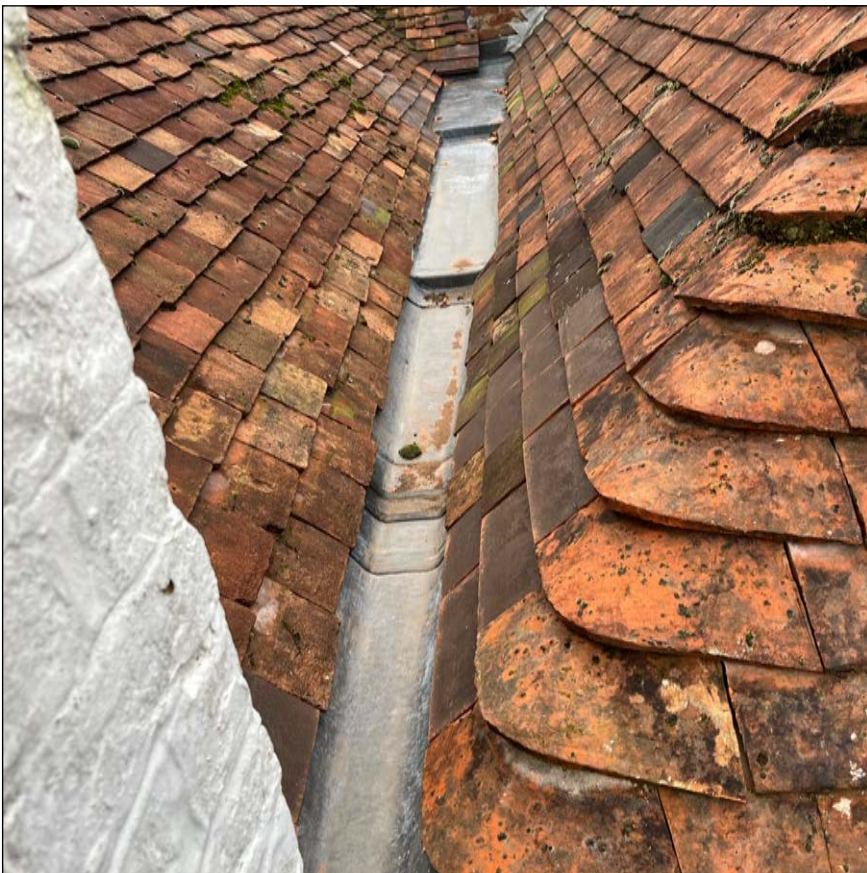
Figure 20: Example of recent roof repairs by the present owner to stop leaking lead gutter and allow ceiling repairs
