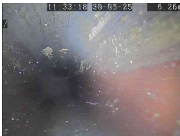
IC1X_be7cd570-4ca7-453f-ac48-1612c56e9c7d_20250604_13 2720_585.jpg, 00:00:20, 6.26 m Line deviates left
