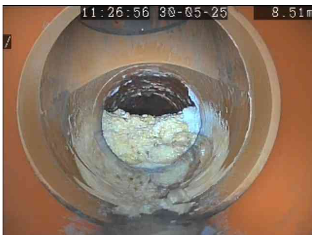
InternalX_c2824007-2947-4b7a-b1c0-2463925ce845_20250604_131439_676.jpg, 00:00:39, 8.60 m Settled deposits, coarse, 50% cross-sectional area loss
