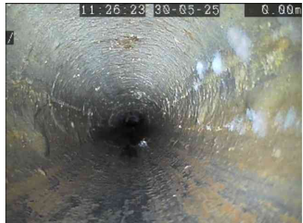
InternalX_d7a14202-124a-4108-900b-8a39d523f016_20250604_131258_732.jpg, 00:00:07, 0.00 m Water level, 5% of the vertical dimension
