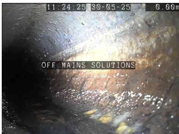
W.C.X_a1dd3d71-662b-4fc3-926e-369a7f08aa7c_20250604_130948_383.jpg, 00:00:00, 3.66 m Finish node, other special chamber, reference: W.C., W.C.
