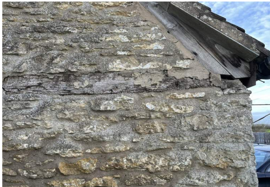
8: Timbers exposed to the elements are soft and have degraded. Stonework would benefit from repointing with lime mortar and locally rebuilding/replacing damaged stones in some locations
