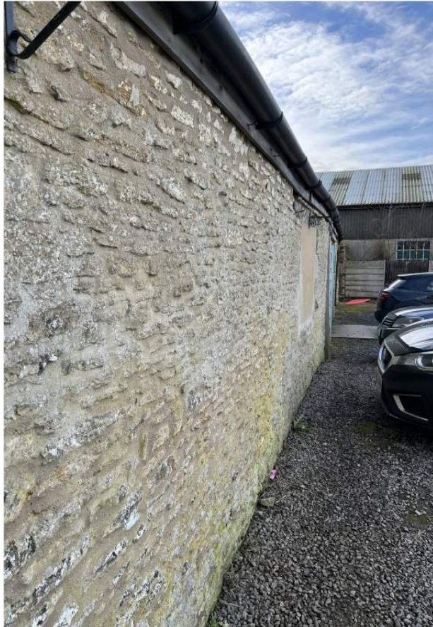
7: Ripples in top of wall reflect areas where the roof has spread
