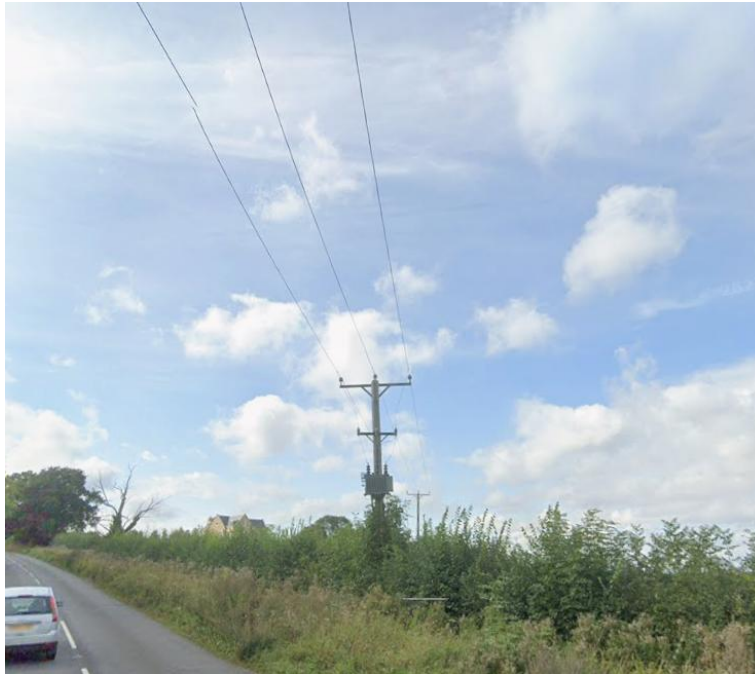
Image 2: Existing 11kV EHV Cables (source Google Earth)
