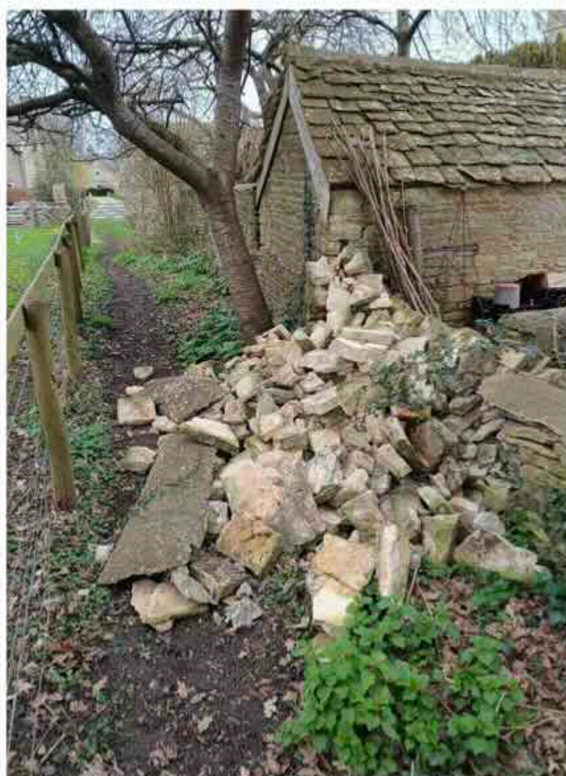
Photo of the garden wall which has collapsed since the Conservation Officers site visit on 03/03/2026
