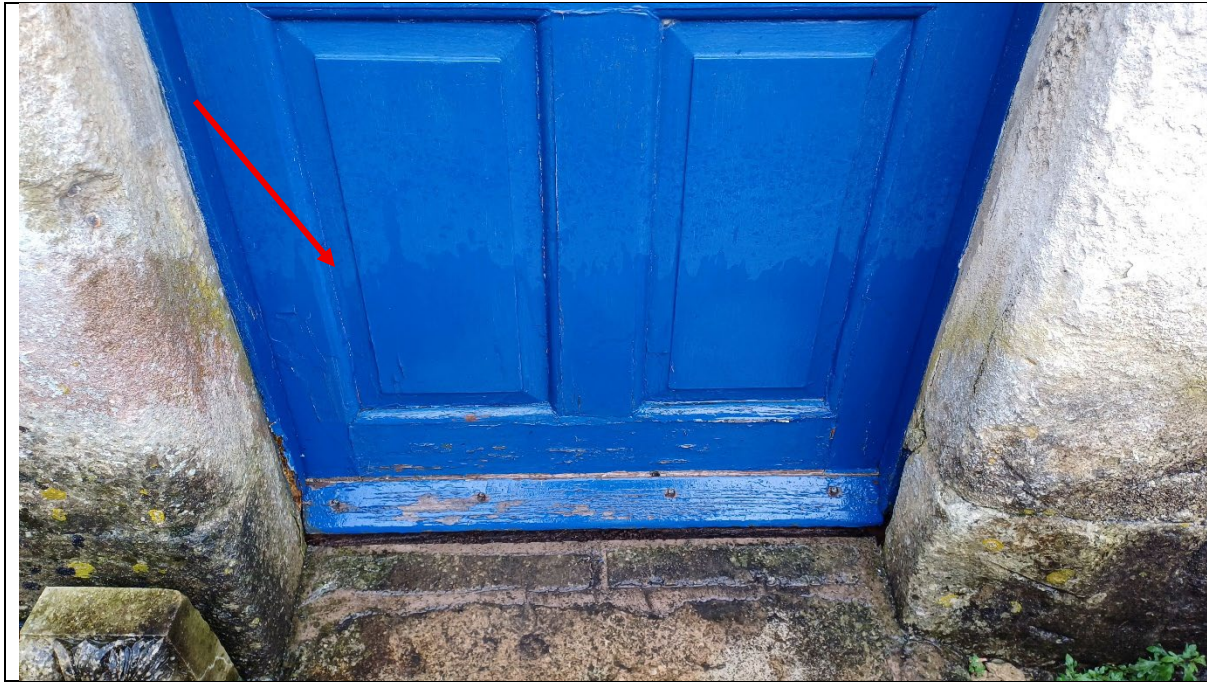
Bottom section of existing door – note height of rainwater splash back
