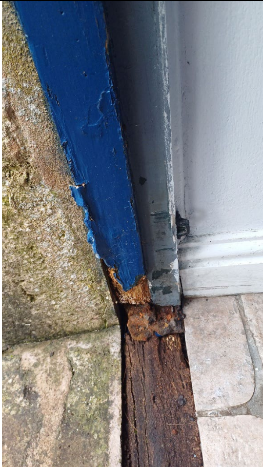
Wood rot at bottom of frame
