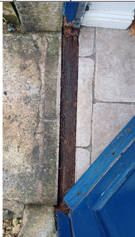
Water-damaged threshold timber
