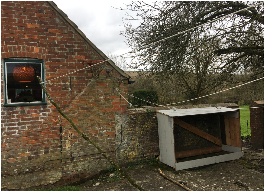
Figure 6 End gable window to be replaced by French windows: with evident Blocking
