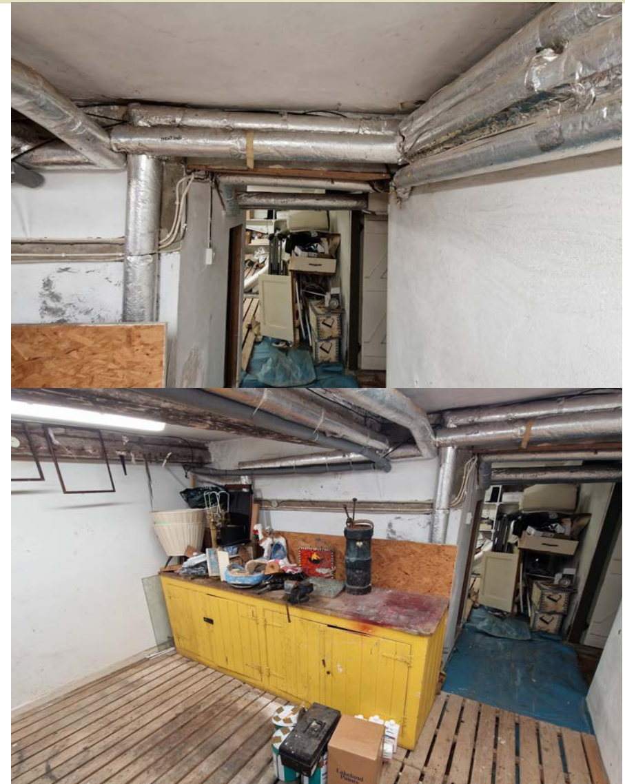
East side with various old boiler pipework
