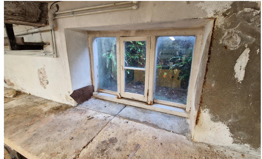
Basement window and wall requiring repair
