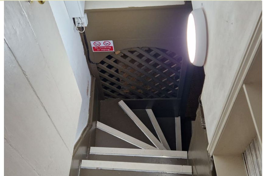
Difficult modern winding stairs to be replaced with safer design
