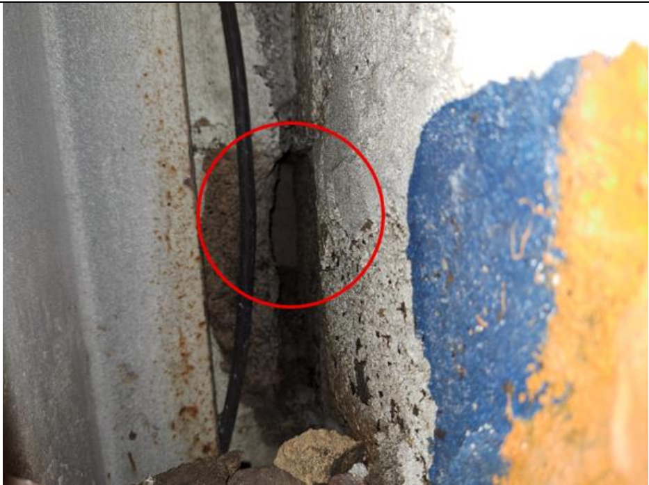
Holes in internal blockwork which appear to lead to a cavity behind the internal and external wall.
