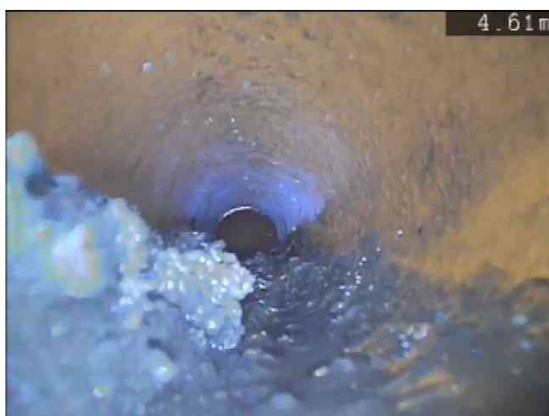
SVP1X_8d2ec630-e787-4dea-bfcf-d6c0afdf1d77_20241206_130526_393.jpg, 00:00:34, 4.61 m Debris, other, 20% cross-sectional area loss, Loose
