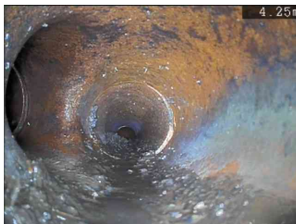
SVP1X_e54b8949-8de3-4482-b53e-6b3516f22f6f_20241206_130454_055.jpg, 00:00:28, 4.25 m Junction at 9 o'clock, 100mm diameter, WG1
