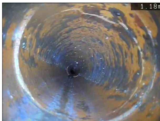
MH1X_ff2fb486-0bd9-4632-926e-02687f8afa35_20241206_130813_761.jpg, 00:00:22, 1.18 m Crack, circumferential at joint from 12 o'clock to 12 o'clock
