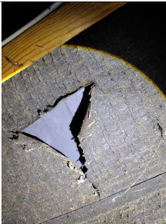
Fig 10. Torn bitumen felt in roof void above link.
