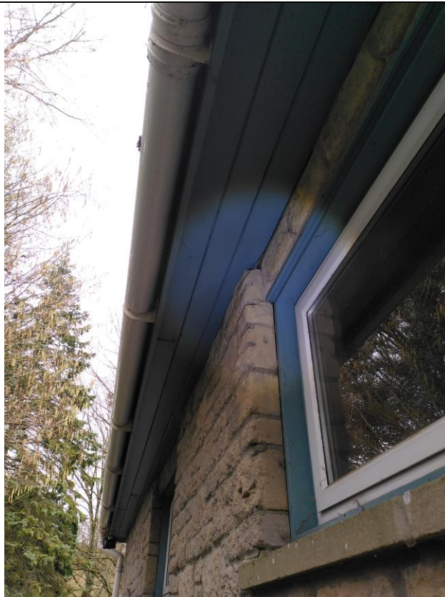
Fig 3. One gap between the brickwork and soffit was also present at the centre of the northeastern elevation
