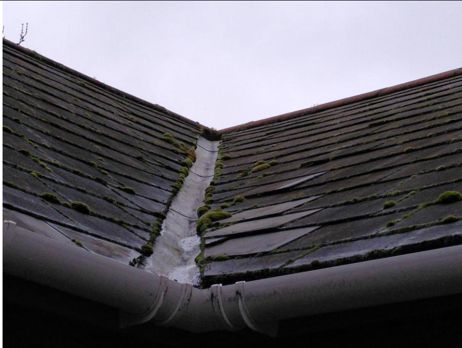
Fig 6. Example of lifted slate tiles.
