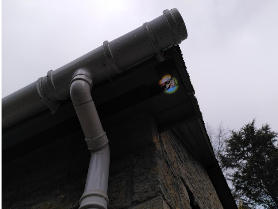
Fig 4. The southern corner hole resulted from some missing venting and evidence of a moss bird nest was present.
