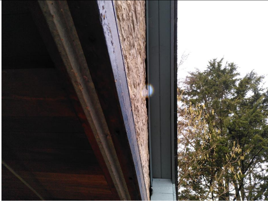
Fig 2. Where the soffit met the stonework on each gable end of the garage there were sufficient gaps to allow bats to enter the garage roof void as well as roost behind the boards themselves.
