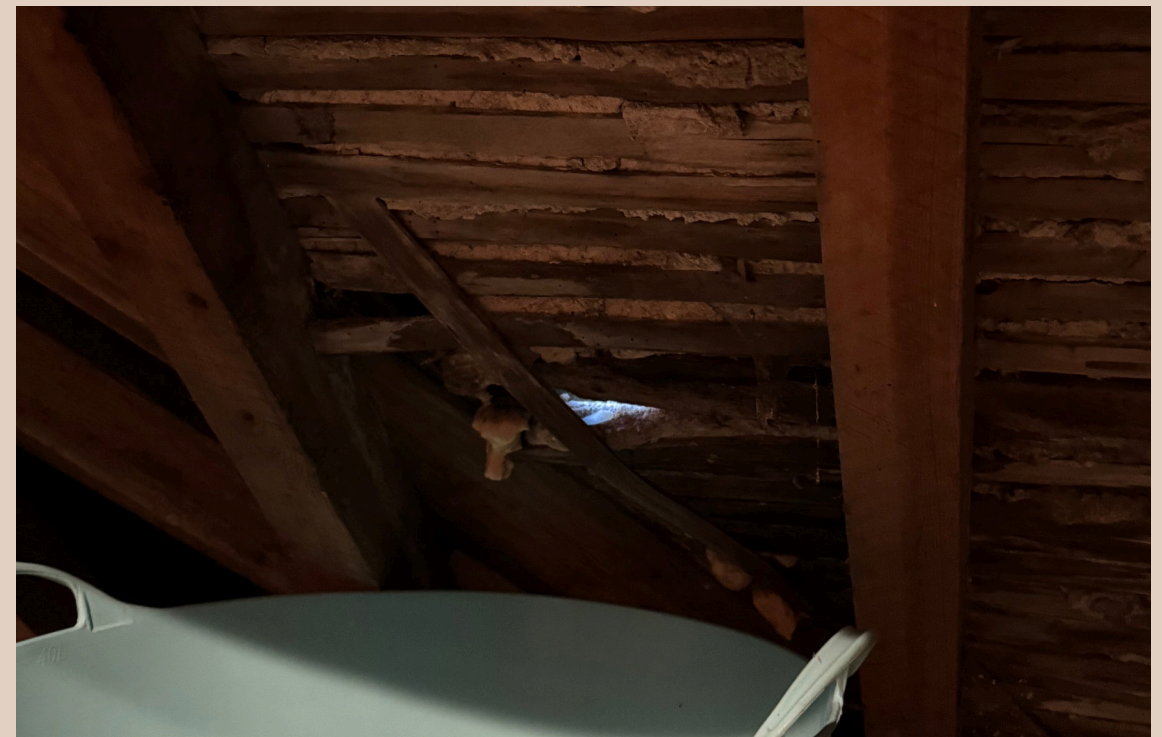
Failing lath & plaster with hole in, this allows water ingress which is damaging ceiling of first floor below.
