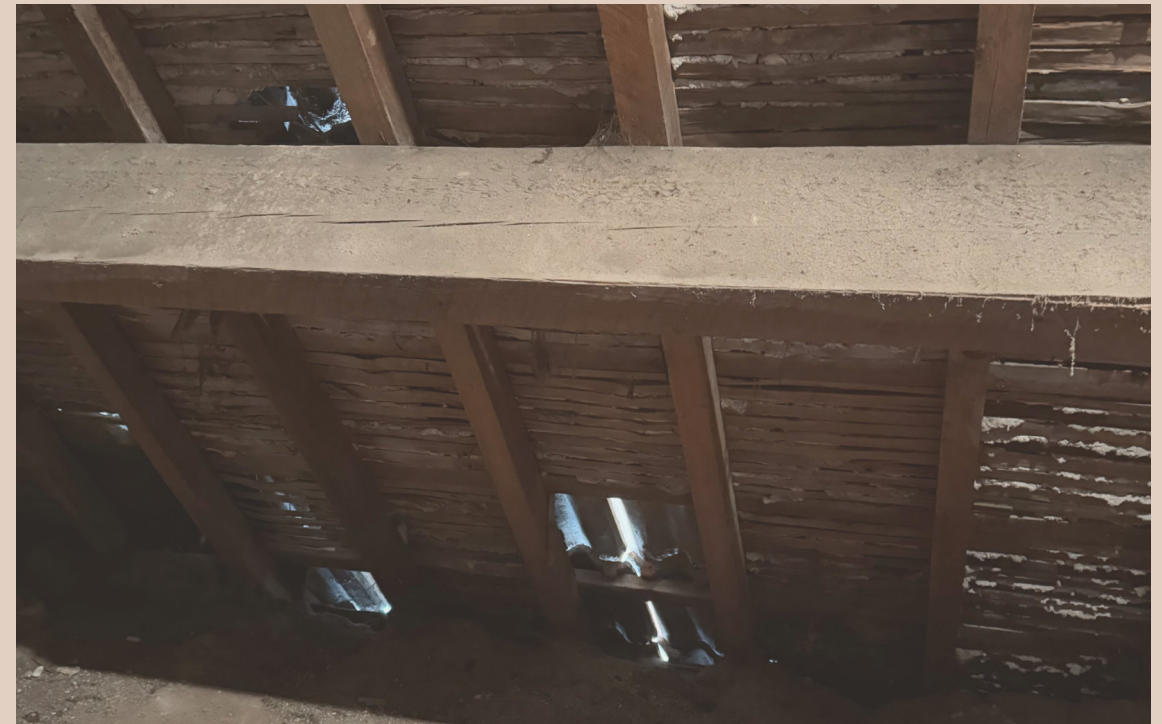
Condition photo of the existing lath & plaster, numerous holes and gaps where the lath and plaster is failing
