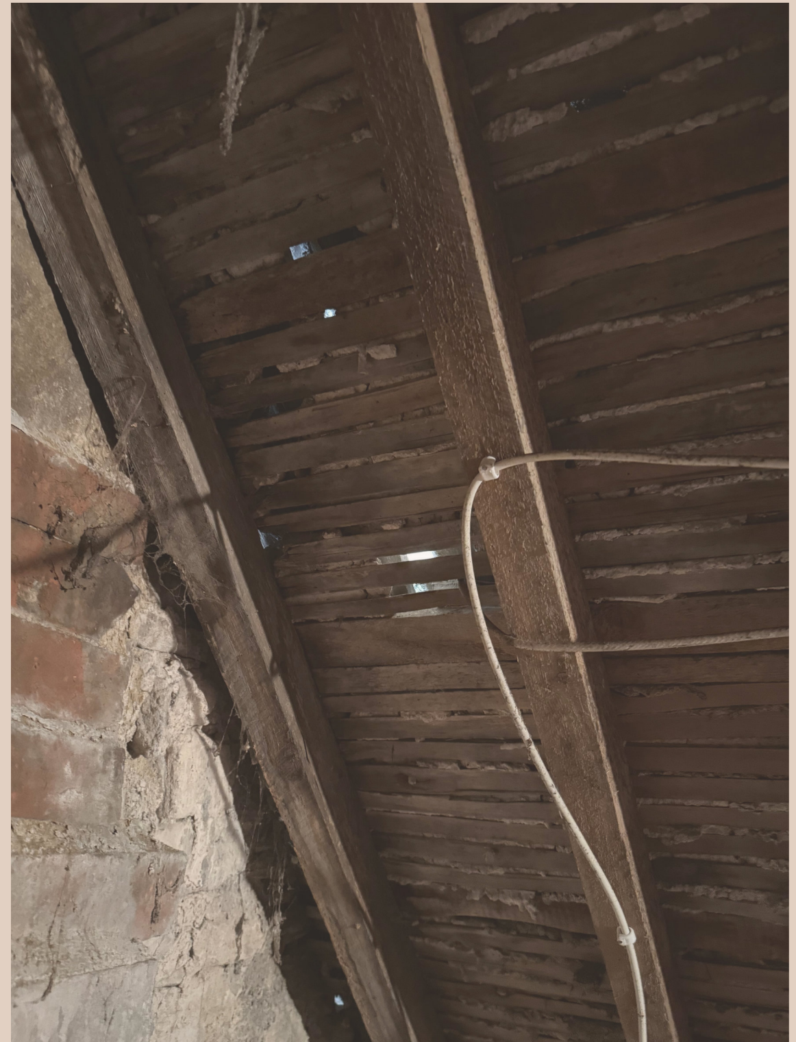
Condition photo of the existing lath & plaster, numerous holes and gaps where the lath and plaster is failing
