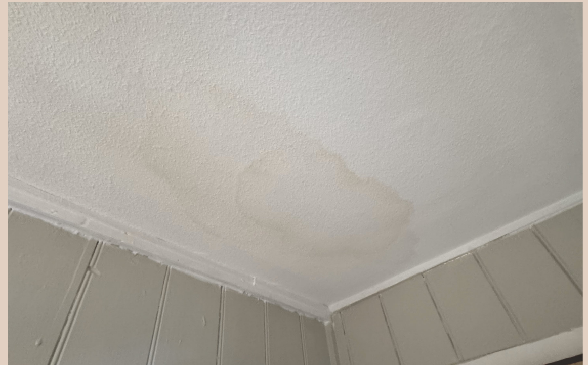
Damage to existing first floor ceiling, caused by failing lath & plaster in roof above.
