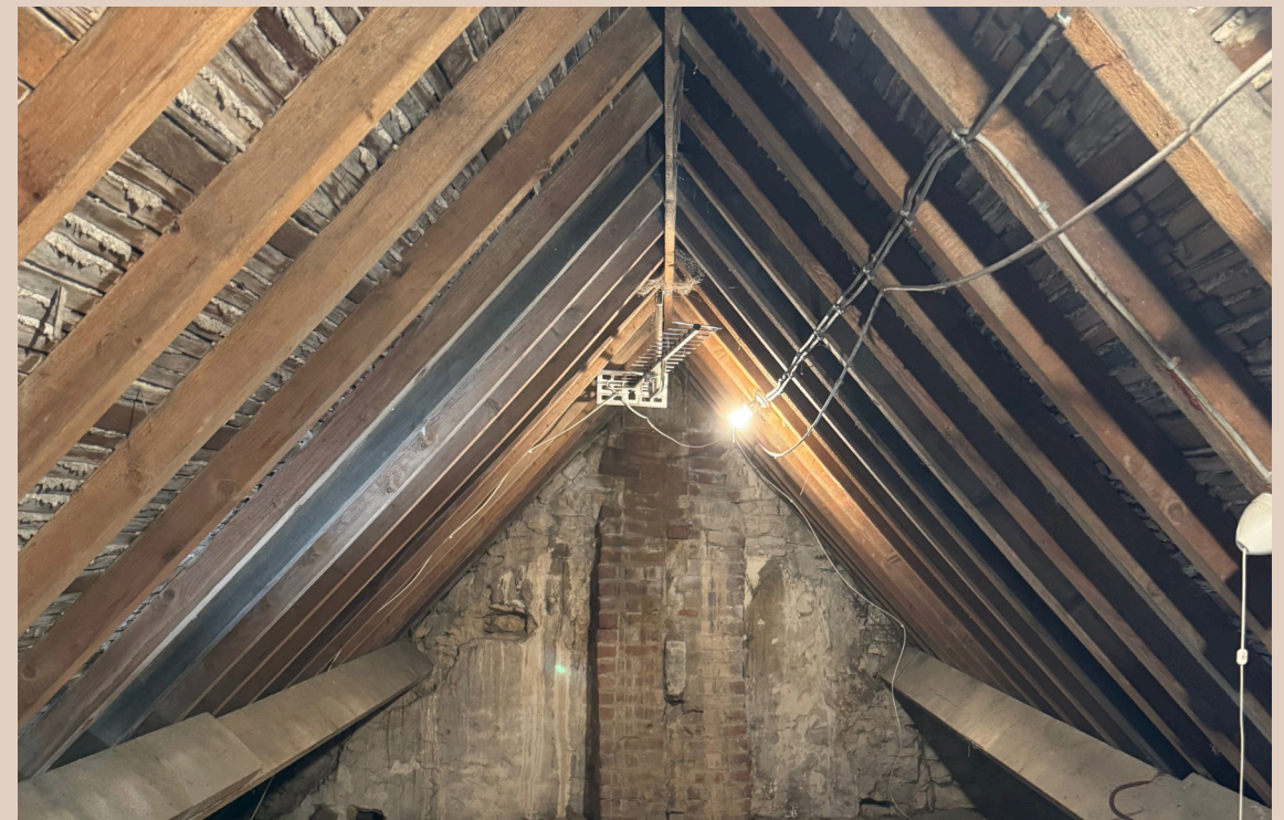
Photo showing the extent of the lath & plaster within the loft space.
