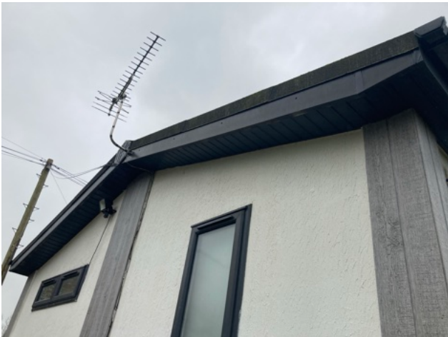
Image 9: Tight soffits, no gaps.
