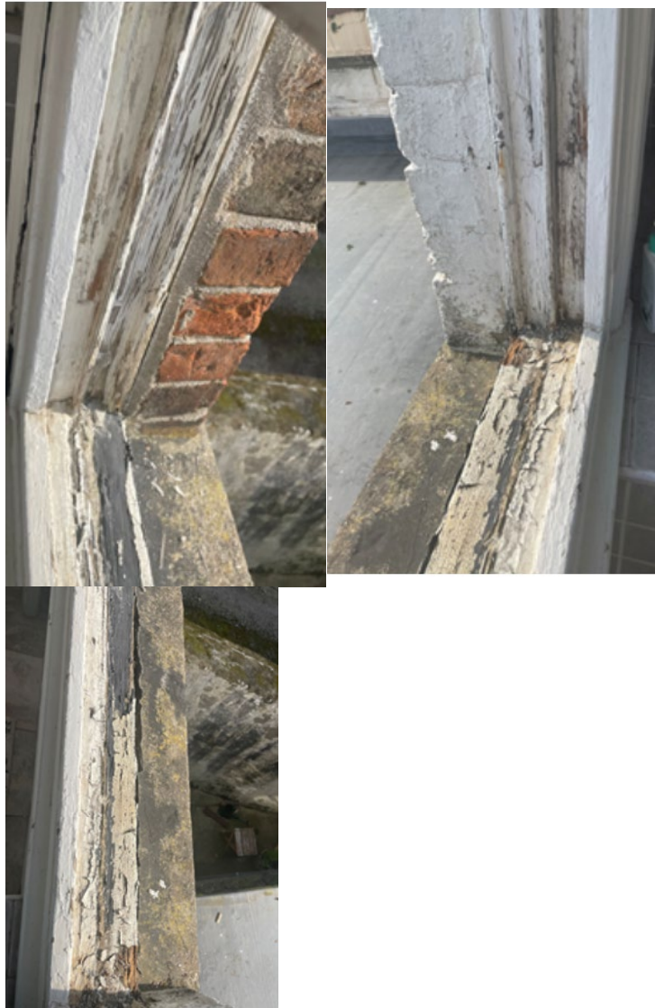
Figure 3 Details of frame showing damage
