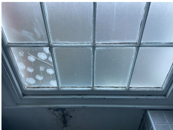
Figure 4 Internal W2 showing damage to lower wall caused by deteriorating frame
