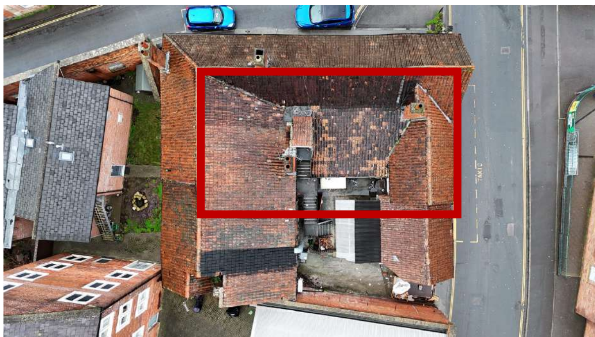
2. View of the roof and areas requiring repair.
