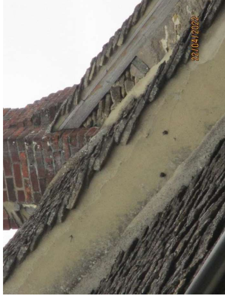
Photo 14: Gaps in the tiles at the verges of the gable ends on the western pitch.
