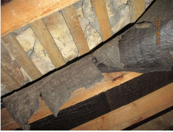
Photo 31: Area of the roof of 'Void 3' where the bitumen lining turns to no lining.
