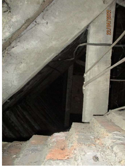
Photo 34: View of Void 4 which was inaccessible.
