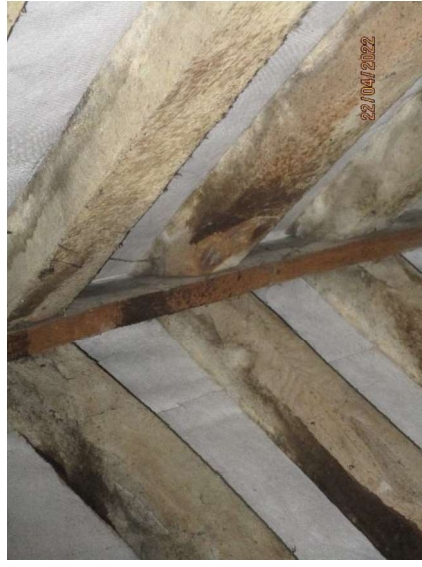
Photo 28: Staining at the ridge beam in 'Void 2'.
