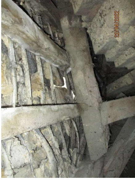
Photo 32: Area of no lining in 'Void 3'.
