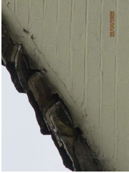
Photo 13: Gaps at the verges at the gable ends of the hotel.
