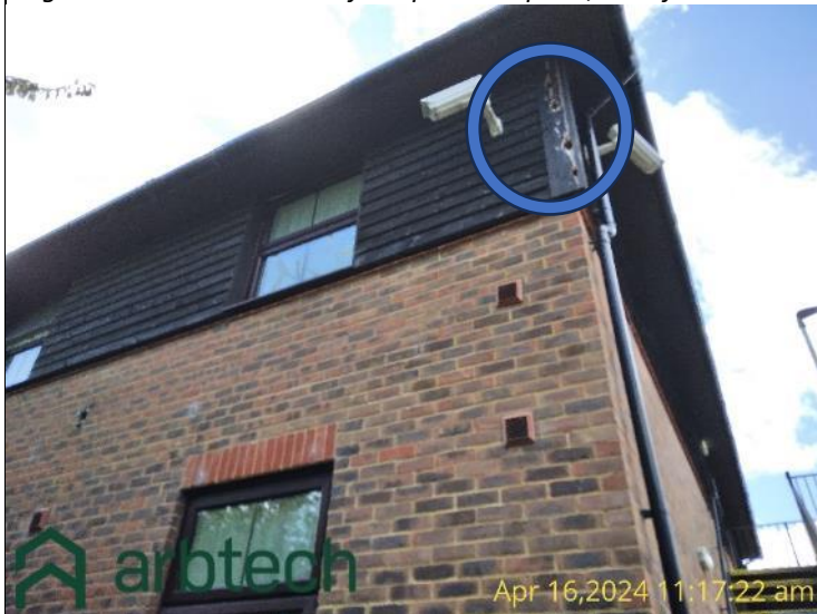
Figure 13- woodpecker holes on the northern corner of B1
