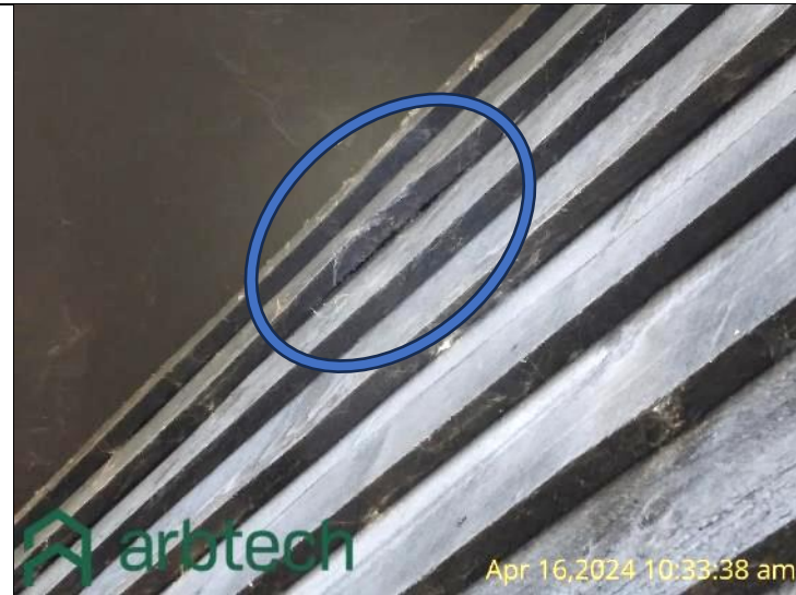
Figure 16- gaps under façade boards on B1 northwest elevation. (circled)
