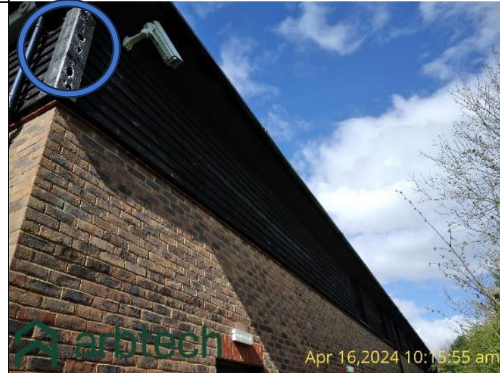
Figure 18- Overall northern view of B1- woodpecker holes in the corner (circled)
