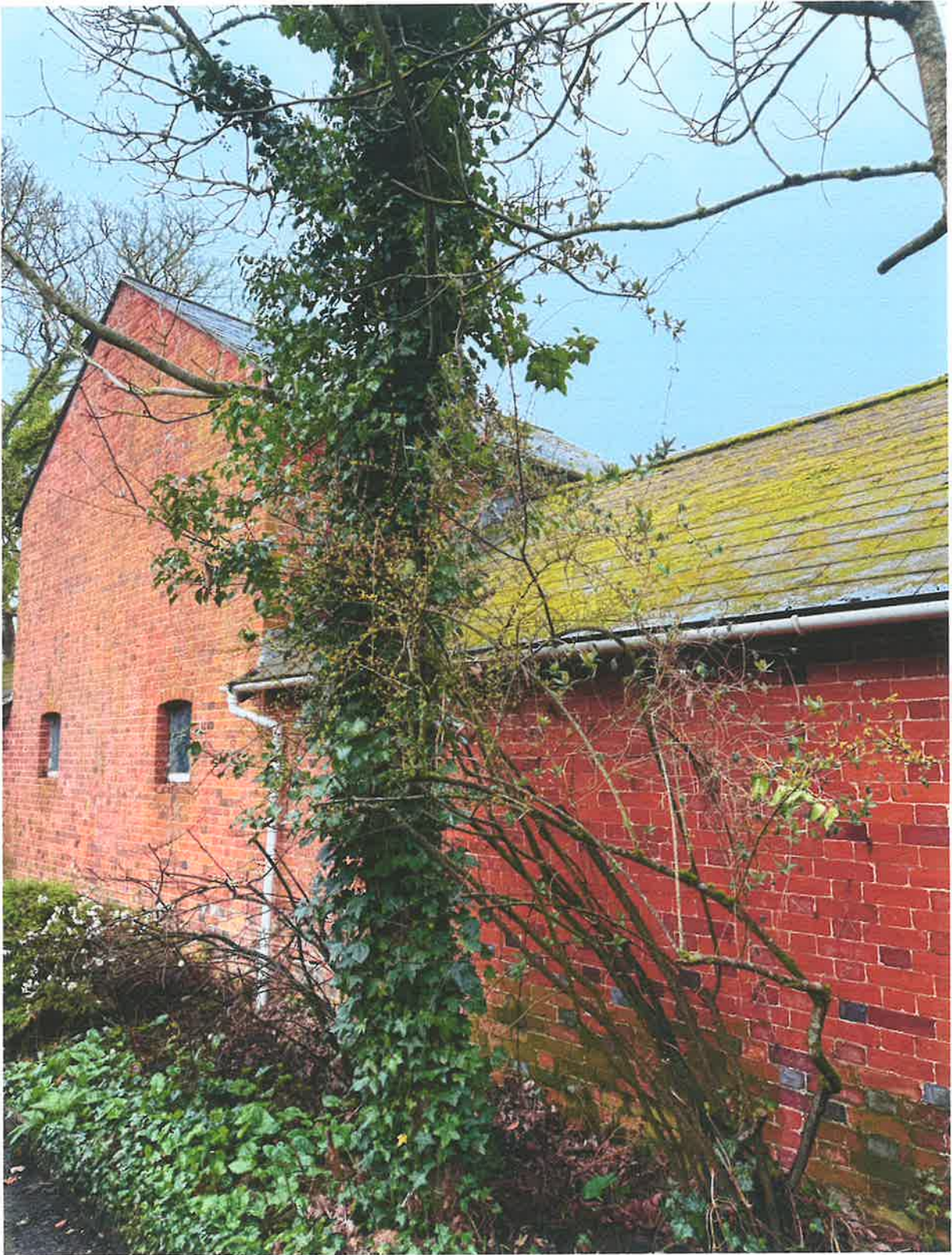
Tree 2 Sapling tree Roots causing damage to Victorian building
