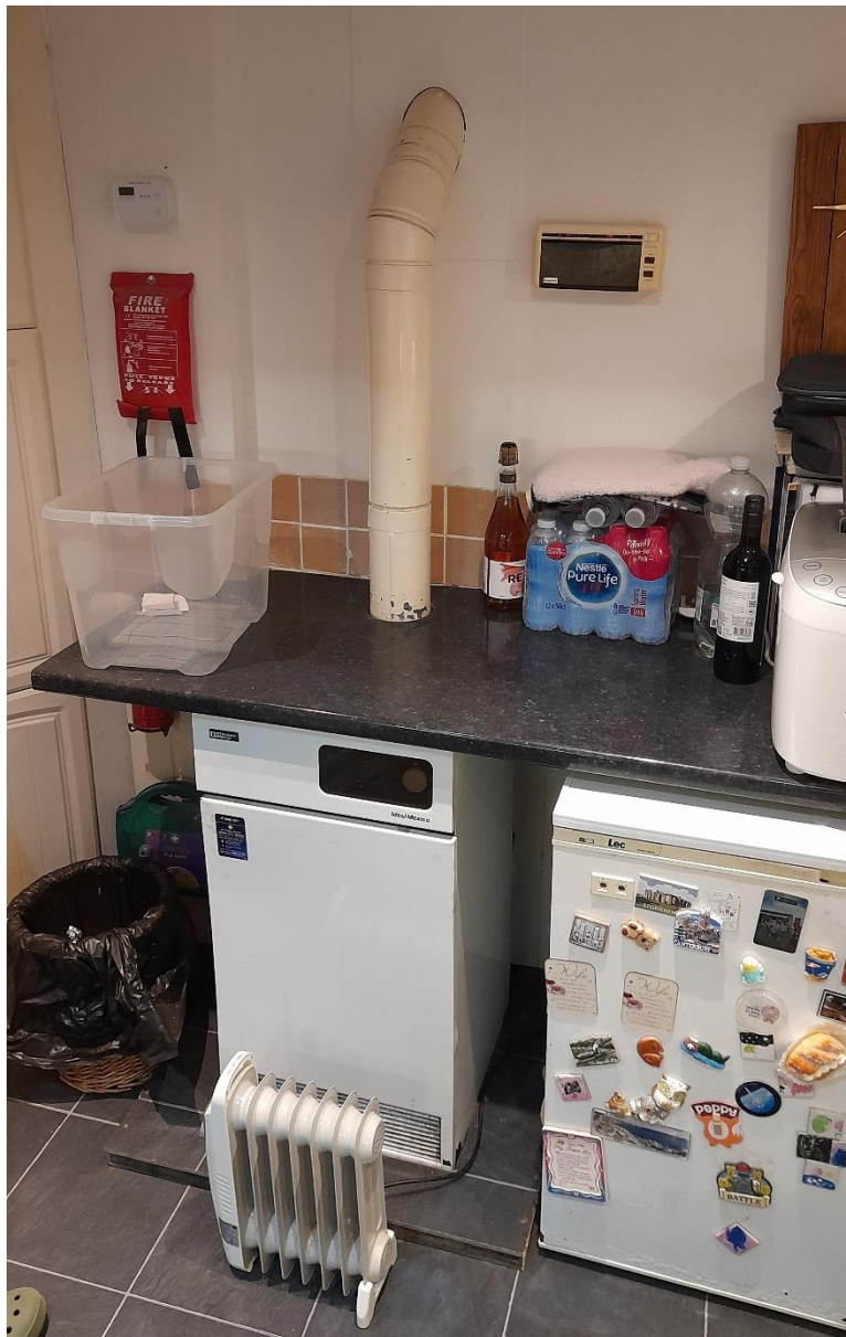
Photograph 2: The existing boiler and existing heating pipework outlet through the wall, which will be reused.
