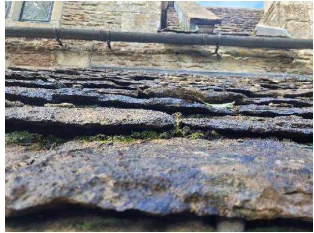
Photograph 20. Stone roof covering with natural gaps offering potential access points for bats.
