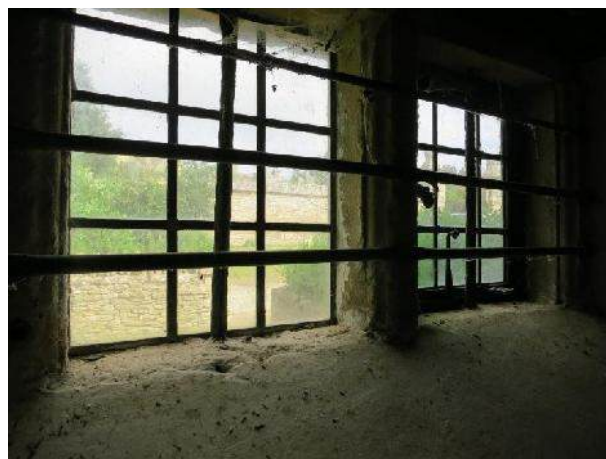
Photograph 28. B13, old bat droppings under the lintel of two windows on the ground floor of the Stables.
