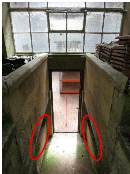
Photograph 48. B5, squash courts with underground voids
