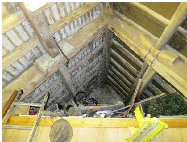
Photograph 27. B13 (Coach House), lime torching under on side of the pitch and bitumen felt on the other side.
