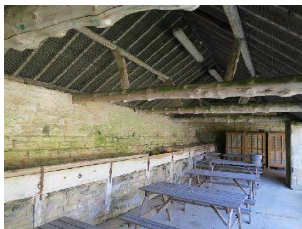
Photograph 32. B11, wire mesh and exposed timbers.
