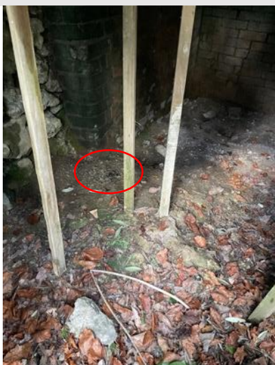
Photograph 9: Entrance to Chamber 5, depicting bat droppings on floor.
