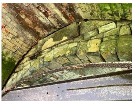
Photograph 14: Depicting shifted stonework above the archway following heavy rain in early 2024 (14 th March 2024).
