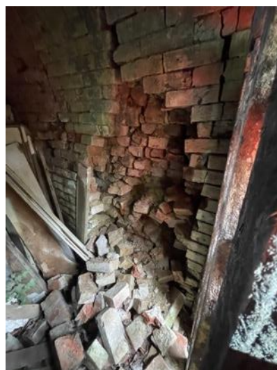
Photograph 18: Depicting shifted brickwork around the doorway to Chamber 4 on the west elevation, following heavy rain in early 2024.
