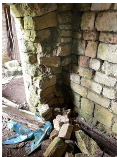
Photograph 16: Depicting shifted stonework around the doorway to Chamber 2, following heavy rain in early 2024.
