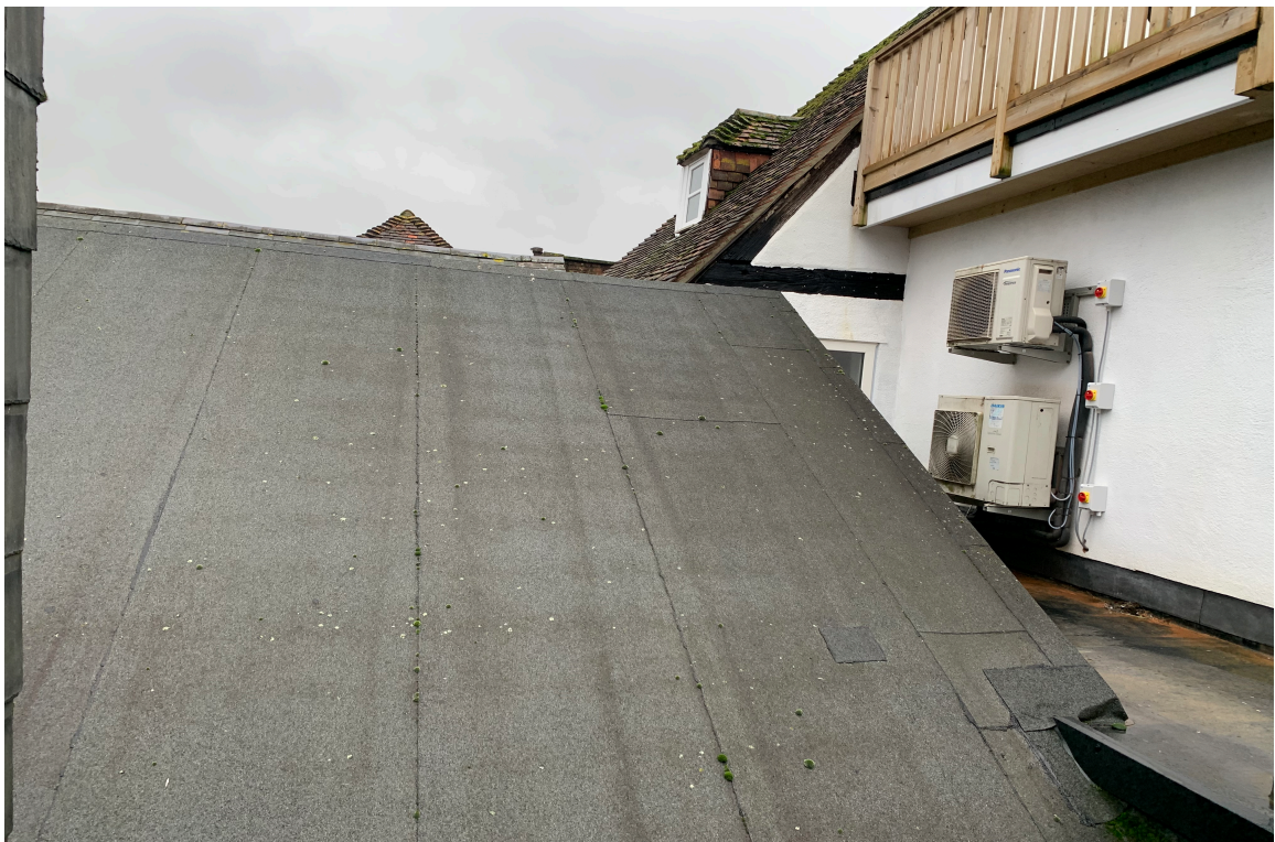
Photo 2, 3 – Roof area and previous repair work
