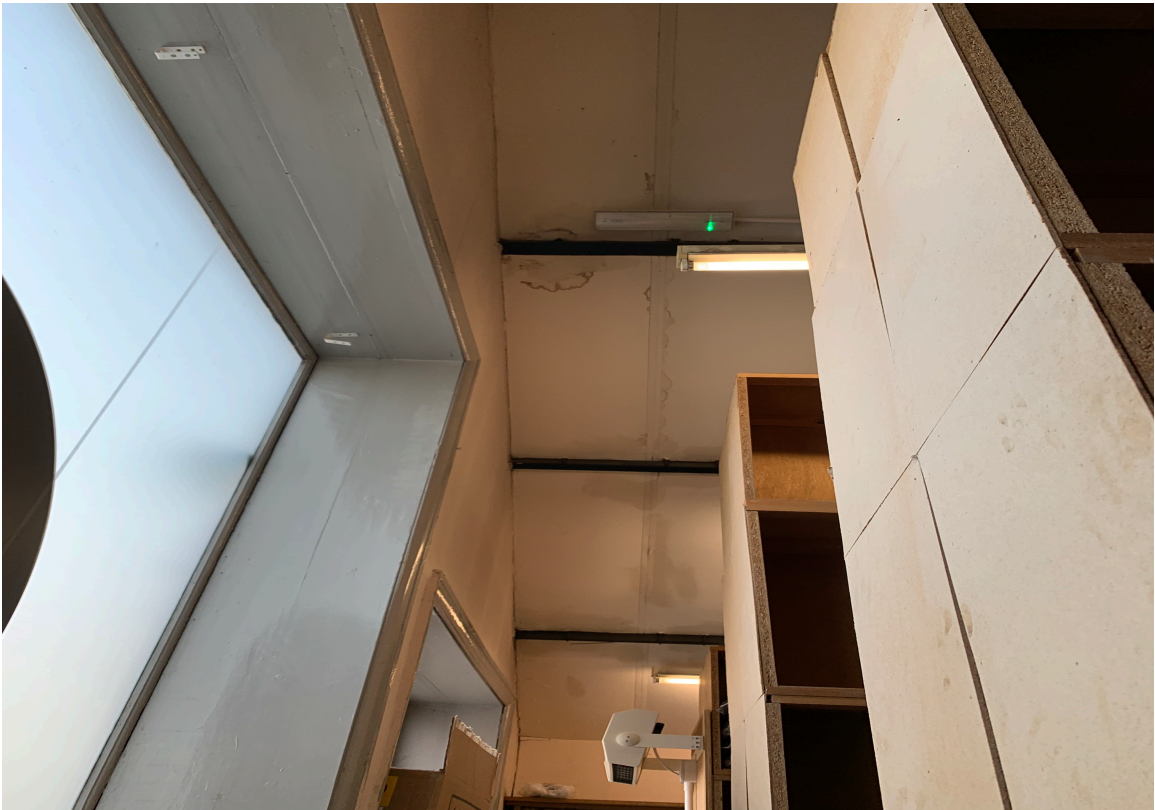
Photo 5, 6 – Evidence of water ingress
