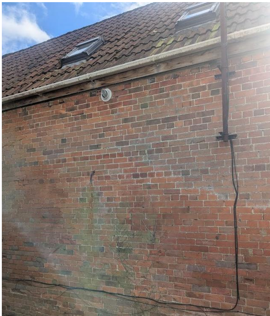
External wiring, rooflights, satellite mount, and boiler vent
