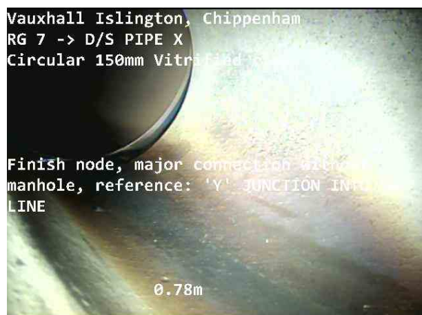
RG 7X_7f445f69-472f-4628-9f4c-de0e15c9c410_20230711_1313 51_293.jpg, 00:00:19, 0.78 m Finish node, major connection without manhole, reference: 'Y' JUNCTION INTO SW LINE
