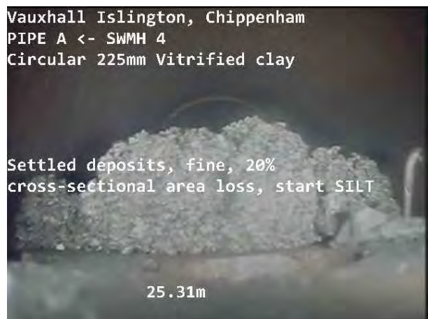
PIPE AX_d120af3a-7c9d-4754-b5c1-ba9839a6e5ec_20230711_094 028_797.jpg, 00:03:20, 25.31 m Settled deposits, fine, 20% cross-sectional area loss, start, SILT
