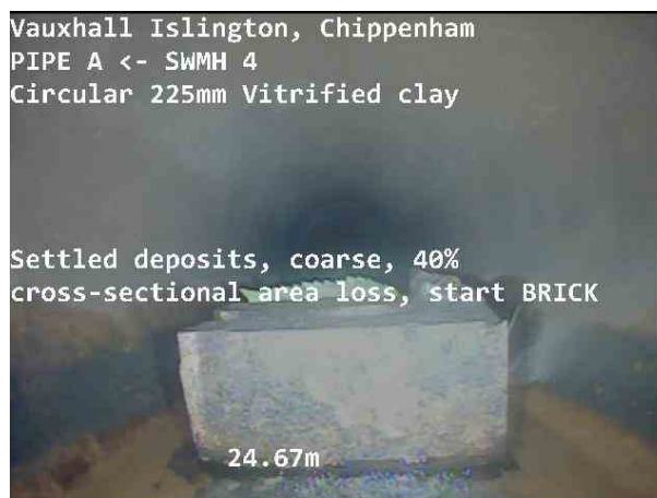
PIPE AX_6fc8e9e3-740a-4102-86c4-426f0b336a1e_20230711_094 013_563.jpg, 00:03:11, 24.67 m Settled deposits, coarse, 40% cross-sectional area loss, start, BRICK
