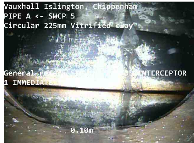
PIPE AX_a3b26e9c-0146-43d9-b800-737662d5798d_20230711_10 1005_430.jpg, 00:00:43, 0.10 m General remark, SERVING PETROL INTERCEPTOR 1 IMMEDIATELY
