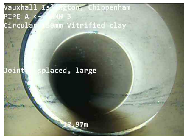
PIPE AX_7a4f39e2-0f79-48ac-87a9-d5776d9bee14_20230711_090 541_359.jpg, 00:03:27, 18.97 m Joint displaced, large
