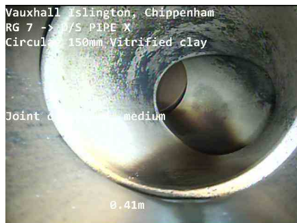
RG 7X_8f0deb33-0d47-4479-8d01-e465d9d885e2_20230711_13 1337_284.jpg, 00:00:11, 0.41 m Joint displaced, medium
