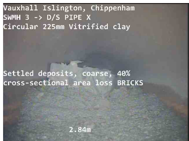
SWMH 3X_0488e0e9-e6ff-43ae-921e-4a4e59d2d454_20230711_115 356_549.jpg, 00:00:31, 2.84 m Settled deposits, coarse, 40% cross-sectional area loss, BRICKS
