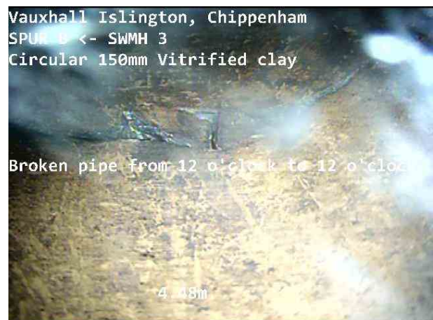
SPUR BX_cf934c93-70ae-4d90-ad09-7e85ffe27bb9_20230711_092 136_393.jpg, 00:01:27, 4.48 m Broken pipe from 12 o'clock to 12 o'clock
