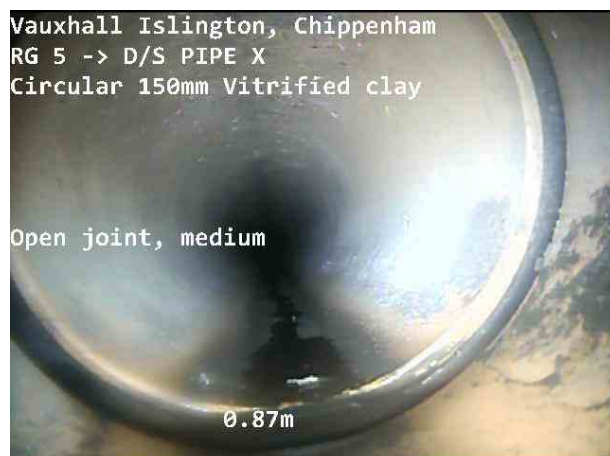
RG 5X_ff808134-c572-4cbf-97f5-804f55946c5c_20230711_13064 6_976.jpg, 00:00:20, 0.87 m Open joint, medium
