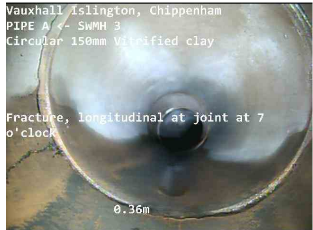
PIPE AX_a1e632f0-205e-4055-a8de-ff3bd7f533a3_20230711_0901 44_674.jpg, 00:00:12, 0.36 m Fracture, longitudinal at joint at 7 o'clock
