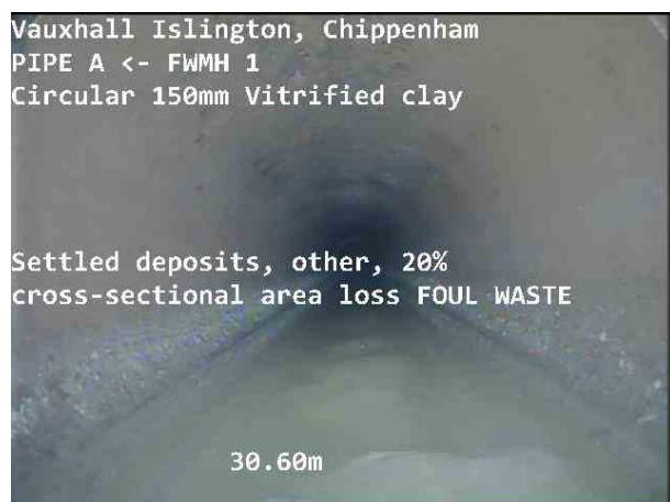
PIPE AX_6fe19d29-b396-4065-b3bd-62a1ca7a5fd0_20230711_111 050_319.jpg, 00:04:15, 30.60 m Settled deposits, other, 20% cross-sectional area loss, FOUL WASTE
