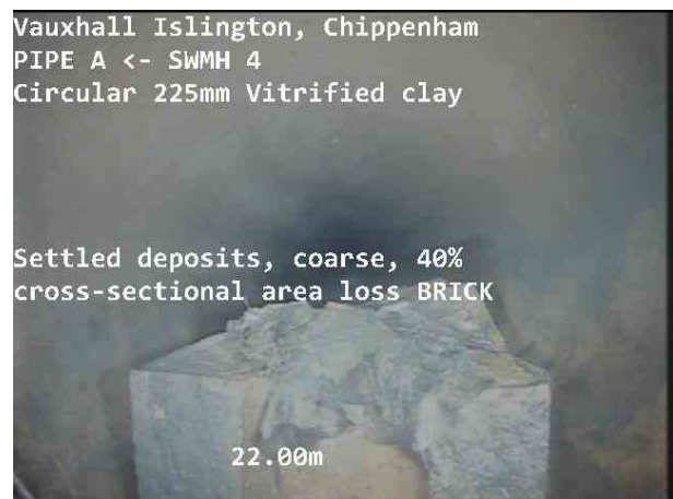
PIPE AX_e1c55dab-d3cc-463b-8430-b706d2846deb_20230711_09 3923_597.jpg, 00:02:37, 22.00 m Settled deposits, coarse, 40% cross-sectional area loss, BRICK
