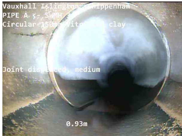
PIPE AX_843bbc85-b821-478d-9976-947ce78e3bf3_20230711_09 0213_145.jpg, 00:00:37, 0.93 m Joint displaced, medium
