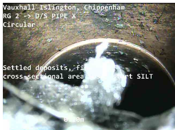
RG 2X_309670b2-69d2-42a6-b533-5c07fdf2fa80_20230711_1248 04_806.jpg, 00:00:03, 0.10 m Settled deposits, fine, 40% cross-sectional area loss, start, SILT
