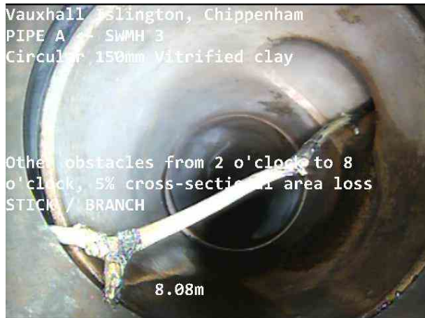
PIPE AX_113974df-d36d-43f5-bd1a-bd3ecbb3eb9a_20230711_090 402_627.jpg, 00:02:00, 8.08 m Other obstacles from 2 o'clock to 8 o'clock, 5% cross-sectional area loss, STICK / BRANCH
