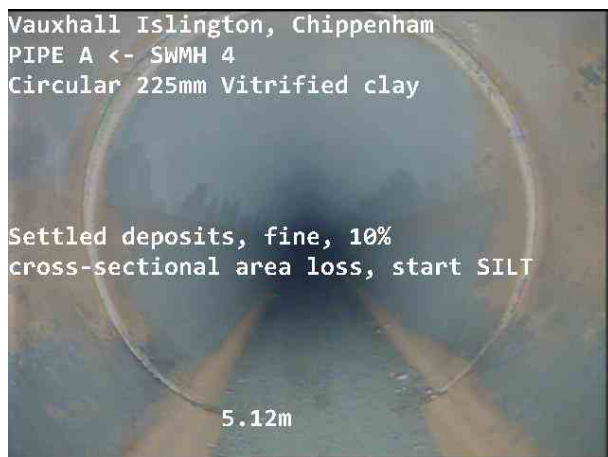
PIPE AX_b5474f41-bc1e-42cb-a929-4a260545c82e_20230711_093 712_357.jpg, 00:00:40, 5.12 m Settled deposits, fine, 10% cross-sectional area loss, start, SILT
