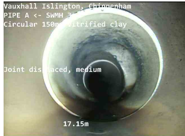
PIPE AX_7d9ab5d1-acc8-4568-bece-d332441ac873_20230711_09 0506_562.jpg, 00:02:59, 17.15 m Joint displaced, medium
