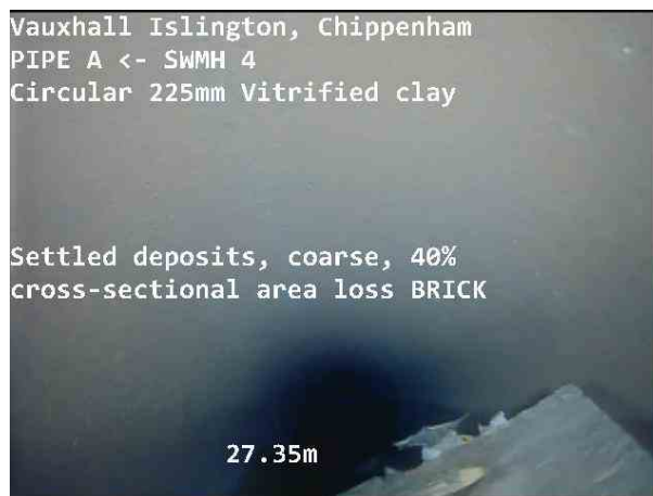
PIPE AX_16c44cb9-5e0d-49be-8582-70ed0682beac_20230711_09 4228_050.jpg, 00:05:18, 27.35 m Settled deposits, coarse, 40% cross-sectional area loss, BRICK
