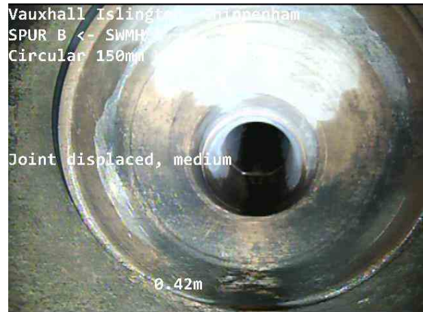
SPUR BX_350fdc2e-91b9-441c-8b68-3a5300e7f937_20230711_092 017_218.jpg, 00:00:22, 0.42 m Joint displaced, medium
