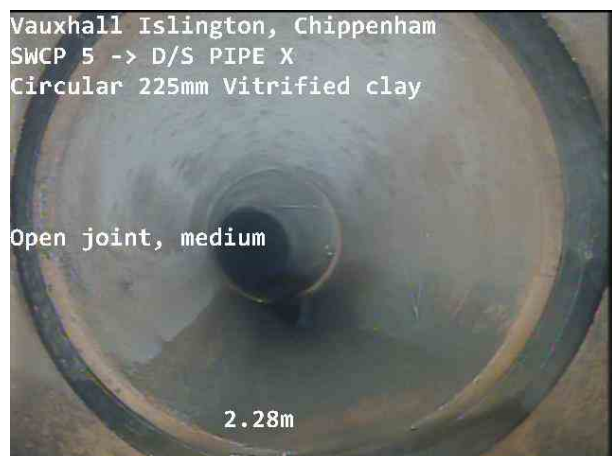
SWCP 5X_e5d70933-cbf0-4ea4-80f0-ce15e169da21_20230711_100 357_098.jpg, 00:00:26, 2.28 m Open joint, medium
