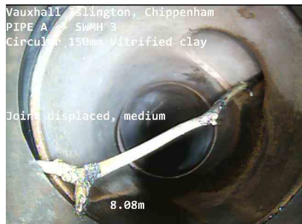
PIPE AX_0c158367-7bde-42d3-94cb-d6a1e6b2959e_20230711_09 0342_281.jpg, 00:01:57, 8.08 m Joint displaced, medium
