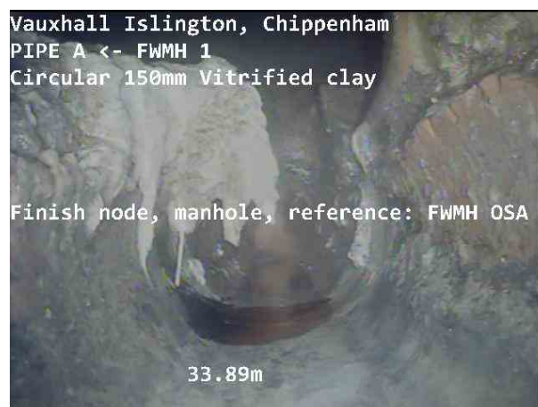
PIPE AX_d343080f-15c8-42ba-9cb9-9c04af8bd3de_20230711_111 302_080.jpg, 00:04:50, 33.89 m Finish node, manhole, reference: FWMH OSA
