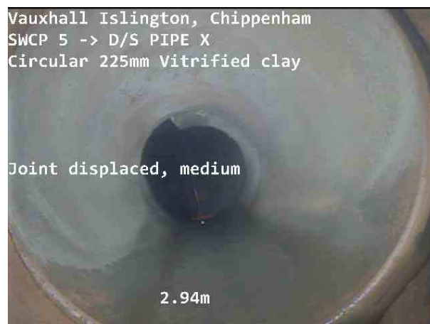
SWCP 5X_7a34d4ff-450e-40a4-aa56-b4e7a41b5278_20230711_100 404_967.jpg, 00:00:34, 2.94 m Joint displaced, medium
