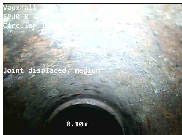
SPUR BX_dca1c935-fbb9-4a61-8f6c-beffd2e2045a_20230711_1140 01_231.jpg, 00:00:05, 0.10 m Joint displaced, medium
