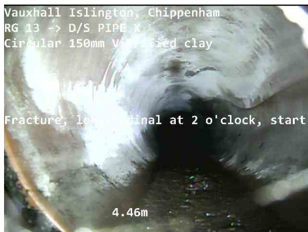
RG 13X_8c3ad9d5-54c1-4fb4-8755-562c4e7fe39b_20230711_13 3641_939.jpg, 00:00:59, 4.46 m Fracture, longitudinal at 2 o'clock, start
