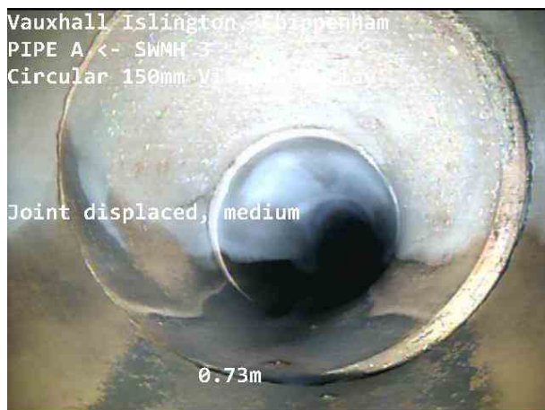
PIPE AX_167758c0-3755-4bb0-928a-8ce73b0cdea6_20230711_09 0159_648.jpg, 00:00:27, 0.73 m Joint displaced, medium
