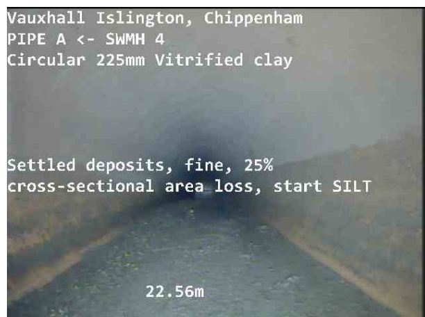
PIPE AX_2ccd8f5e-795d-4678-829f-10b7ca168ee8_20230711_093 947_040.jpg, 00:02:55, 22.56 m Settled deposits, fine, 25% cross-sectional area loss, start, SILT
