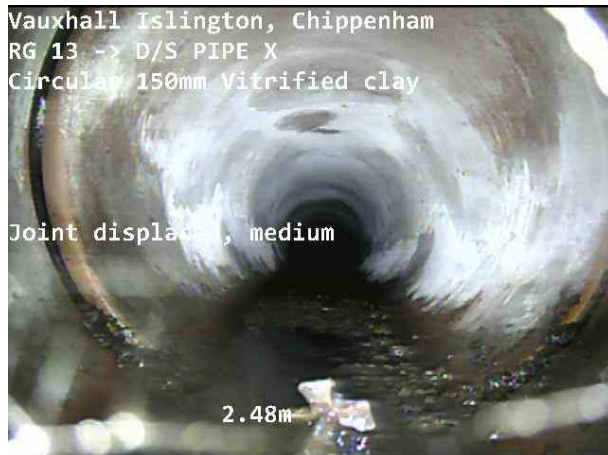
RG 13X_890d517a-9948-4287-bbe3-600ec4bef55e_20230711_13 3611_540.jpg, 00:00:34, 2.48 m Joint displaced, medium
