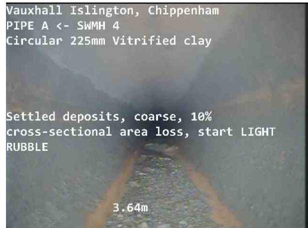
PIPE AX_64c8fd16-aaa4-47c3-ac9f-7efa9d595c77_20230711_0936 54_340.jpg, 00:00:27, 3.64 m Settled deposits, coarse, 10% cross-sectional area loss, start, LIGHT RUBBLE
