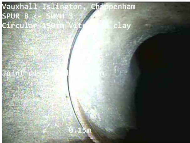
SPUR BX_87d8c37f-e128-46f3-bbec-b437c6904cda_20230711_092 001_285.jpg, 00:00:12, 0.15 m Joint displaced, medium
