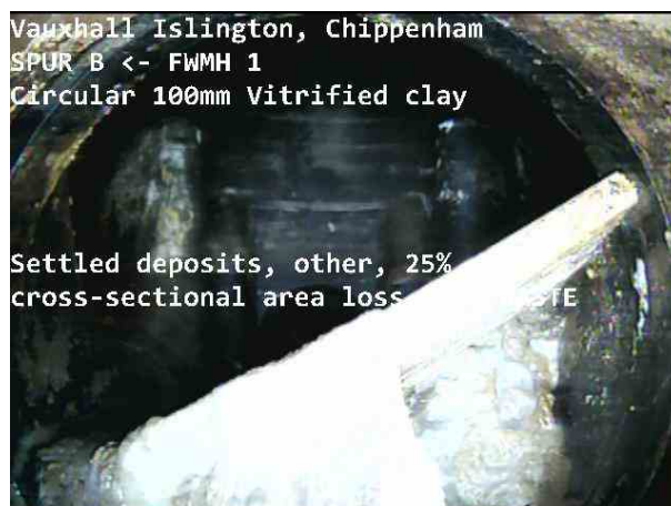
SPUR BX_ce6a6299-99aa-4807-ac95-1b56c28afb65_20230711_114 230_928.jpg, 00:02:20, 15.31 m Settled deposits, other, 25% cross-sectional area loss, FOUL WASTE
