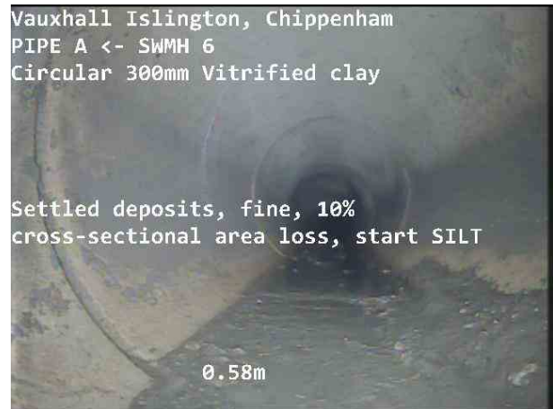
PIPE AX_cbdb87c8-a49a-4bdb-897b-a53288136828_20230711_10 1746_142.jpg, 00:00:08, 0.58 m Settled deposits, fine, 10% cross-sectional area loss, start, SILT
