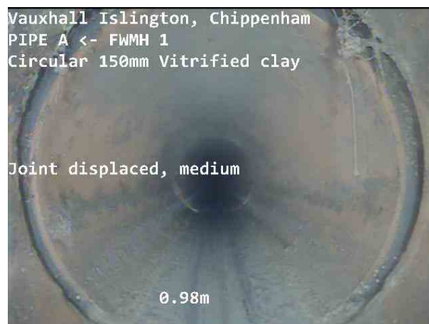
PIPE AX_e4f18a4c-b6a7-4b70-bb2a-c9b58876dd70_20230711_11 0638_624.jpg, 00:00:09, 0.98 m Joint displaced, medium
