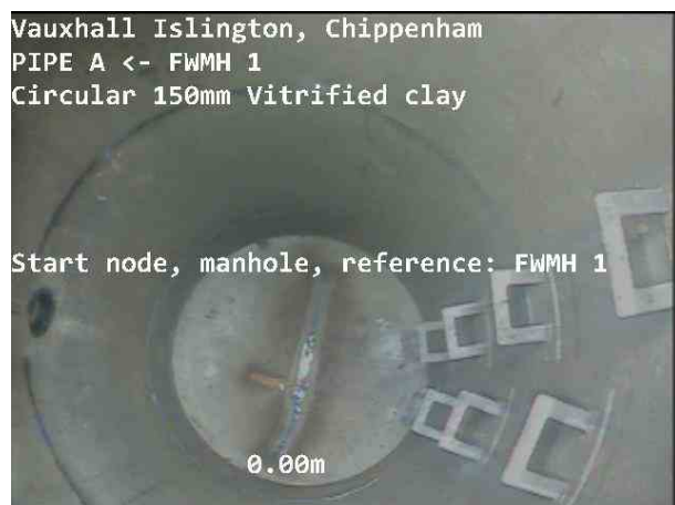
PIPE AX_5029cbdc-2ebf-4e2c-8141-472185aa03df_20230711_110 405_847.jpg, 00:00:00, 0.00 m Start node, manhole, reference: FWMH 1
