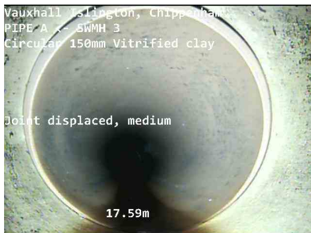
PIPE AX_57133d66-65f5-47b0-b1af-6d29d390ecb5_20230711_090 525_462.jpg, 00:03:13, 17.59 m Joint displaced, medium
