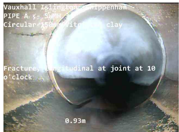
PIPE AX_857c3d95-366a-41c5-b2d7-ef10a96d79f5_20230711_090 210_926.jpg, 00:00:36, 0.93 m Fracture, longitudinal at joint at 10 o'clock
