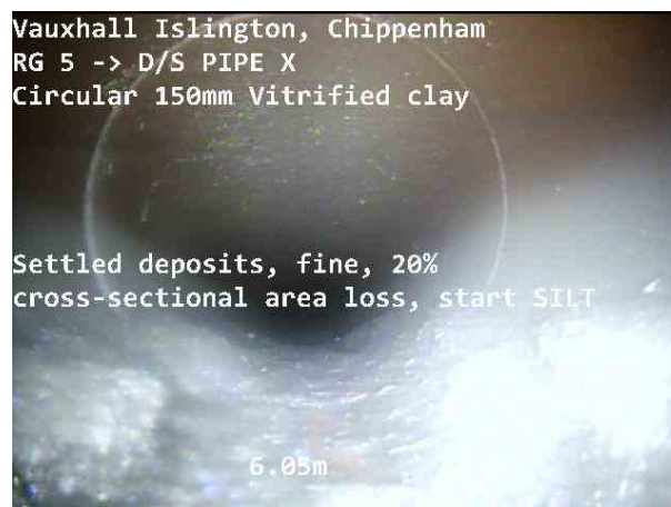
RG 5X_236327e6-7a0e-4091-a543-bf893336ae71_20230711_13 0742_245.jpg, 00:01:13, 6.05 m Settled deposits, fine, 20% cross-sectional area loss, start, SILT
