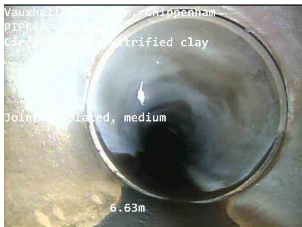
PIPE AX_abcd7673-f29c-48c5-b608-fb885ca1ef48_20230711_0903 25_058.jpg, 00:01:42, 6.63 m Joint displaced, medium
