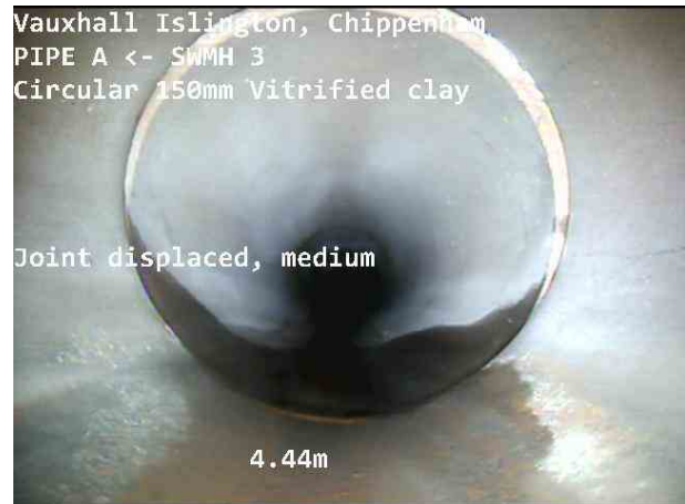
PIPE AX_091f7b32-6f8b-4c7e-8b46-43305dd7cdca_20230711_090 249_473.jpg, 00:01:11, 4.44 m Joint displaced, medium
