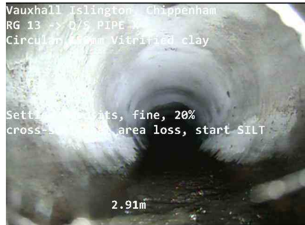
RG 13X_ca4506c2-7a44-4af4-8585-e011bf81d016_20230711_13 3620_217.jpg, 00:00:41, 2.91 m Settled deposits, fine, 20% cross-sectional area loss, start, SILT
