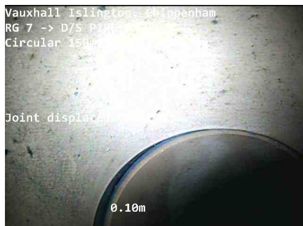
RG 7X_1aabccaa-1892-4ea9-a602-c629aacdf725_20230711_131 327_216.jpg, 00:00:02, 0.10 m Joint displaced, medium
