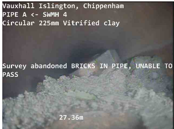
PIPE AX_7678432f-7895-4313-ac17-252942dde95a_20230711_09 4310_627.jpg, 00:05:40, 27.36 m Survey abandoned, BRICKS IN PIPE, UNABLE TO PASS
