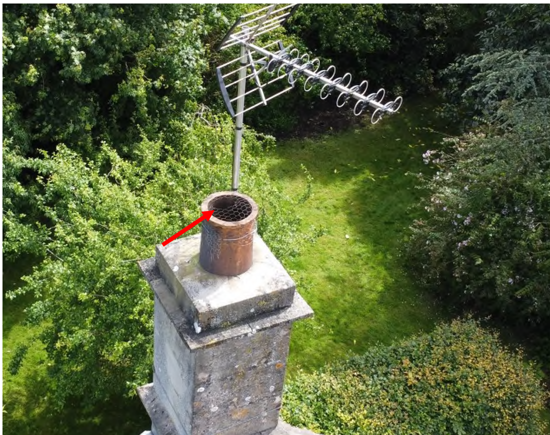
Plate 12 Rip in chicken wire allowed access for jackdaws
