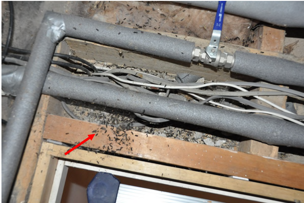
Plate 7 Evidence of bat droppings spilling through the from the underfelt
