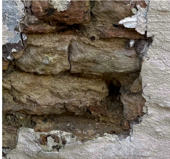
Example of fractured stone most likely caused by expansion of water trapped in the fabric
