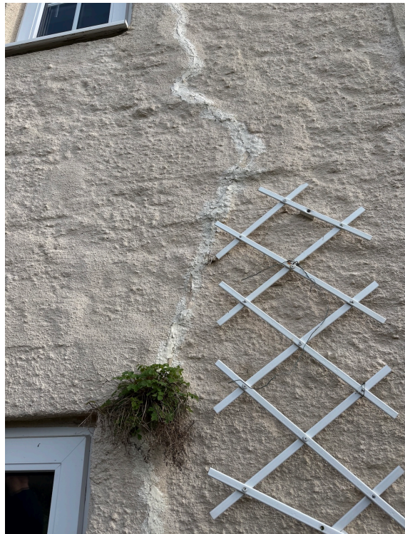
Cracks in the external render with plant growth
