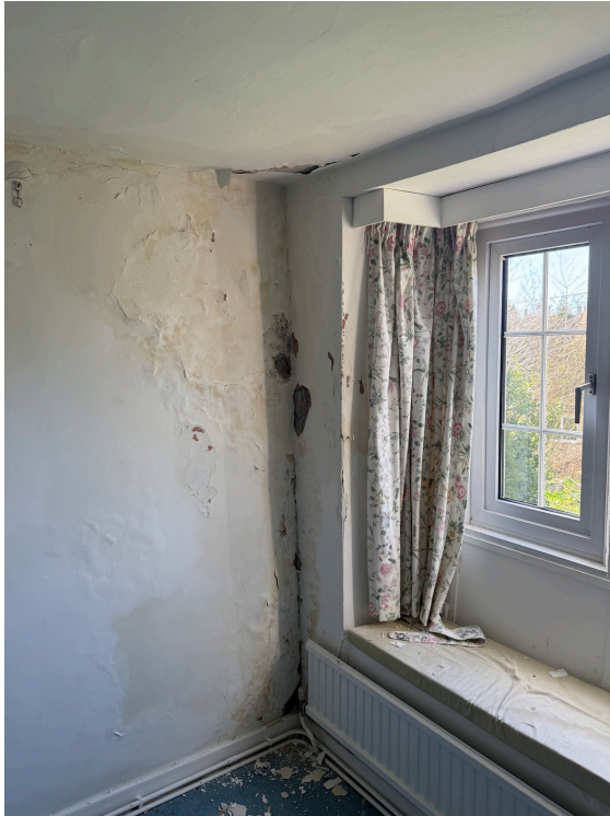
Excessive damp on internal walls
