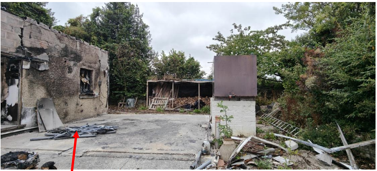
Fire damaged boot room entrance, garage and utility room
