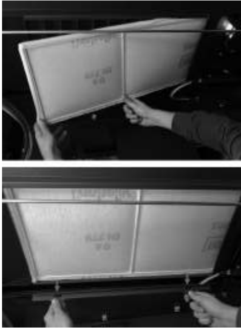
Figure 82: Replacement filter mats
